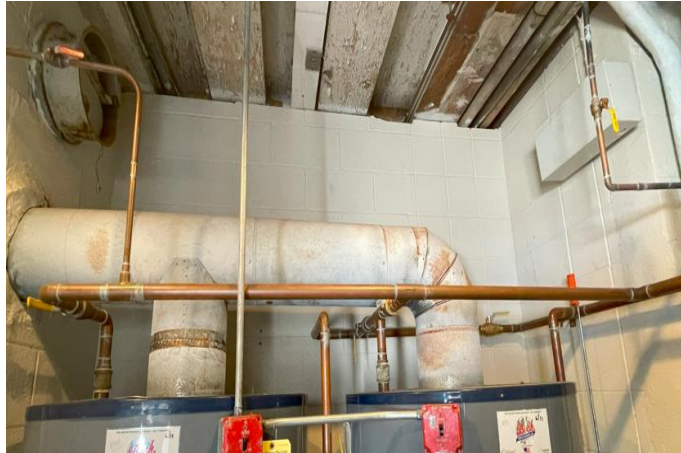
Uninsulated DHW Pipes
