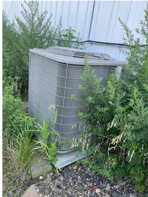
Carrier Condensing Unit Split System
