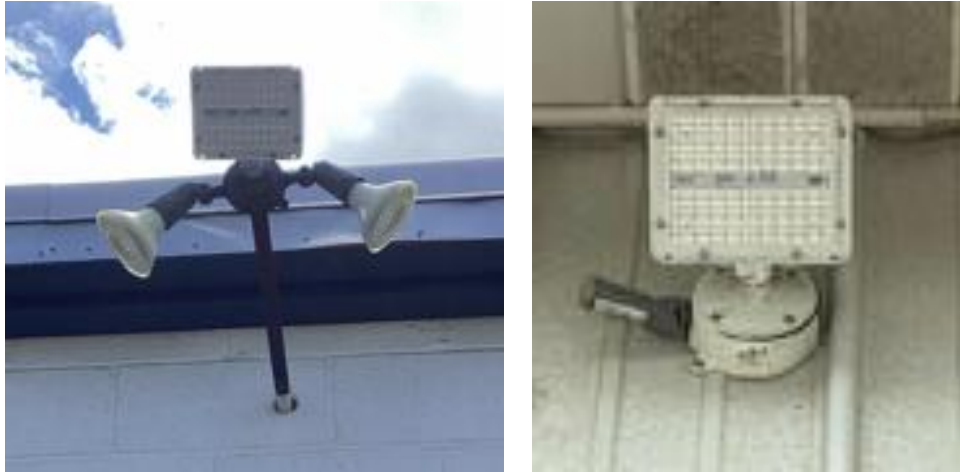
Exterior LED Fixtures
