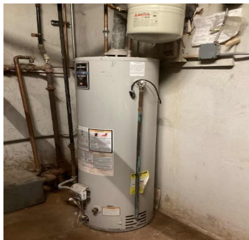
Bradford White DHW Heater
