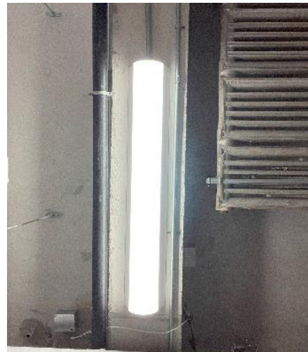
LED 4-foot Fixtures
