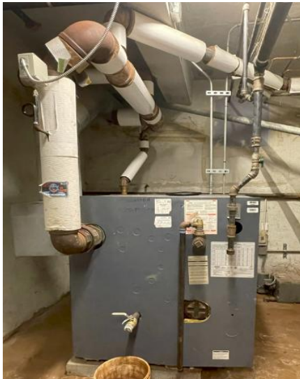
Weil McLain Steam Boiler
