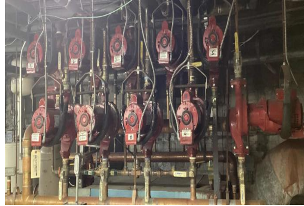
Heating Hot Water Pumps
