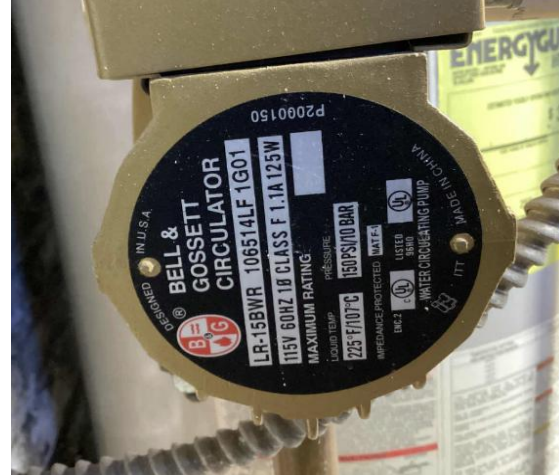
DHW Circulation Pump
