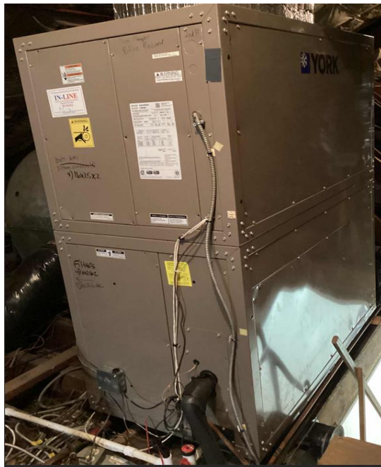
Attic York AHU
