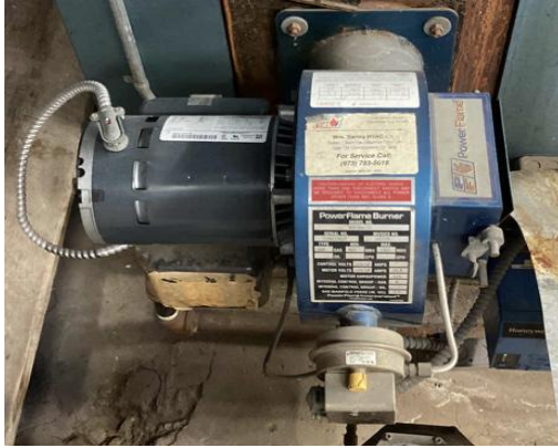
Boiler Combustion Air Fan
