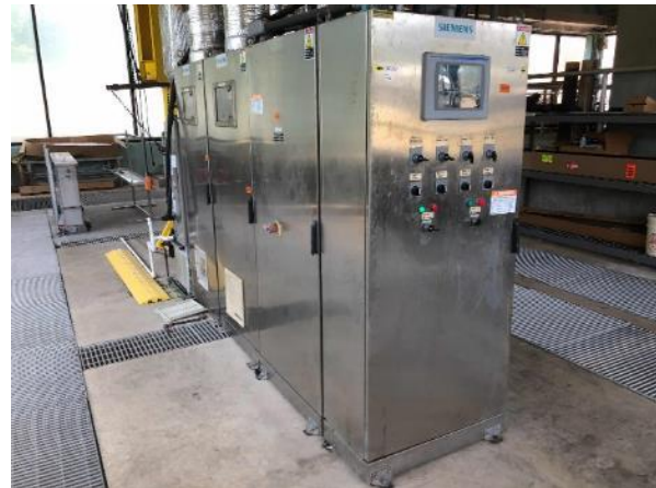
UV Lighting Controls
