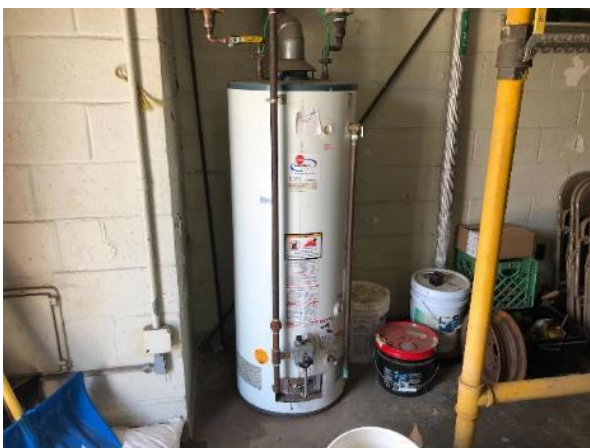
Hot Water Storage Unit
