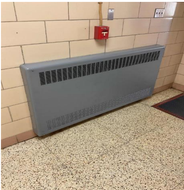
Typical Corridor Hydronic Unit Heater
