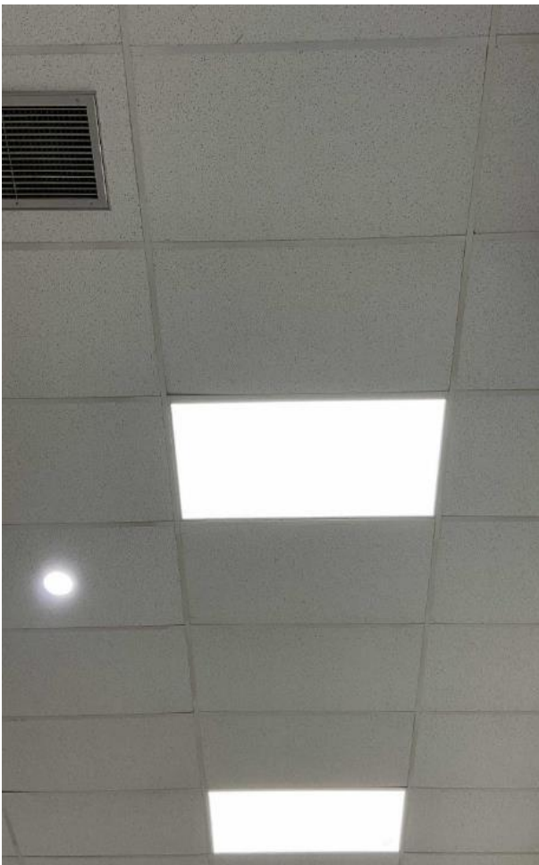
Gymnasium LED Fixtures
