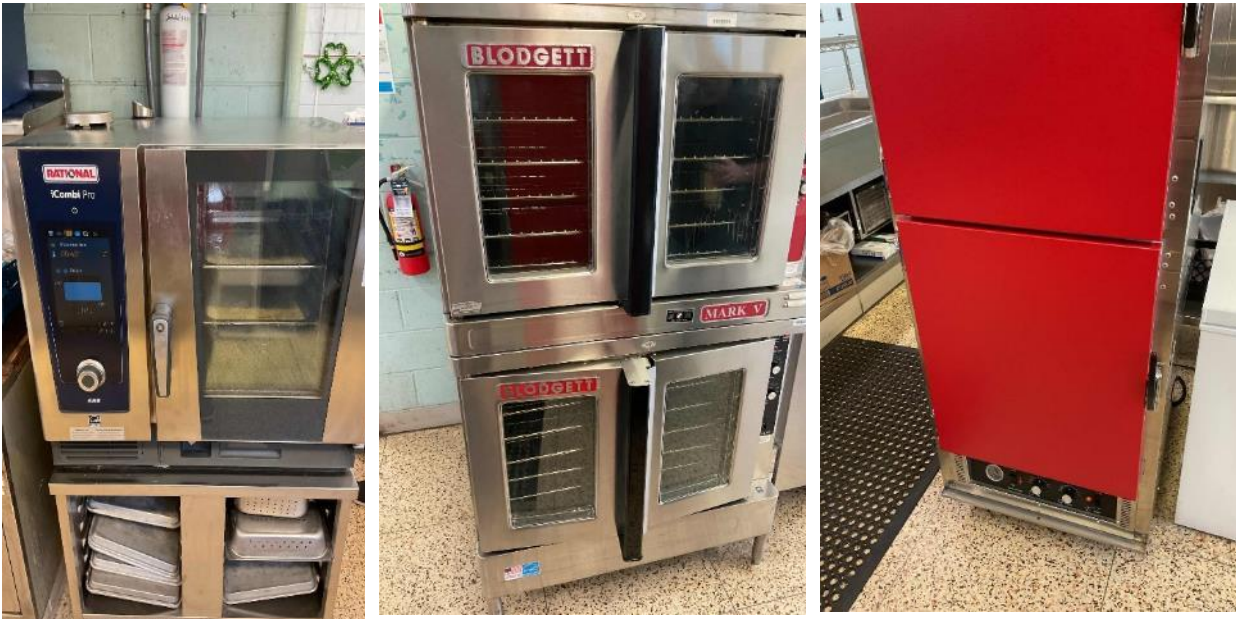
Typical Kitchen Equipment
