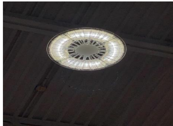
Multipurpose Room LED Fixture
