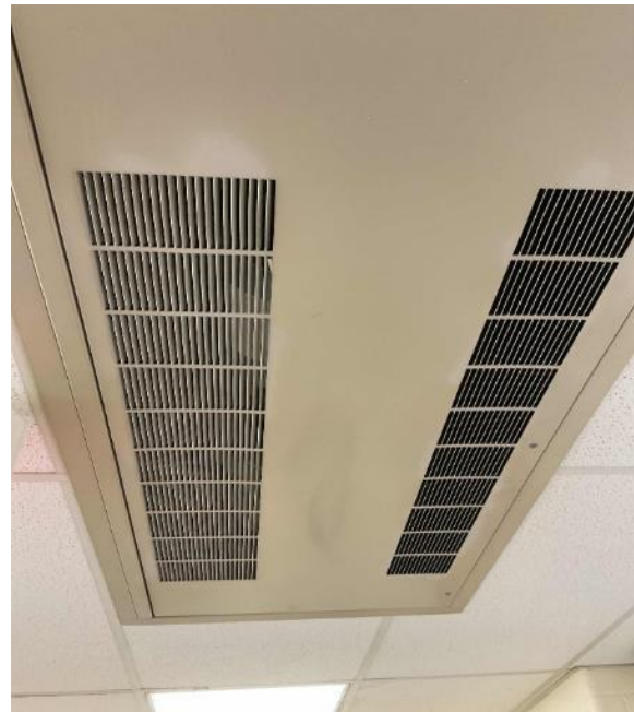
Corridor Unit Ventilators
