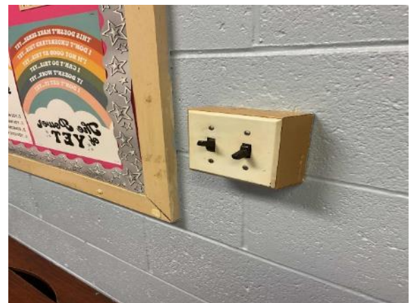
Typical Wall Switch
