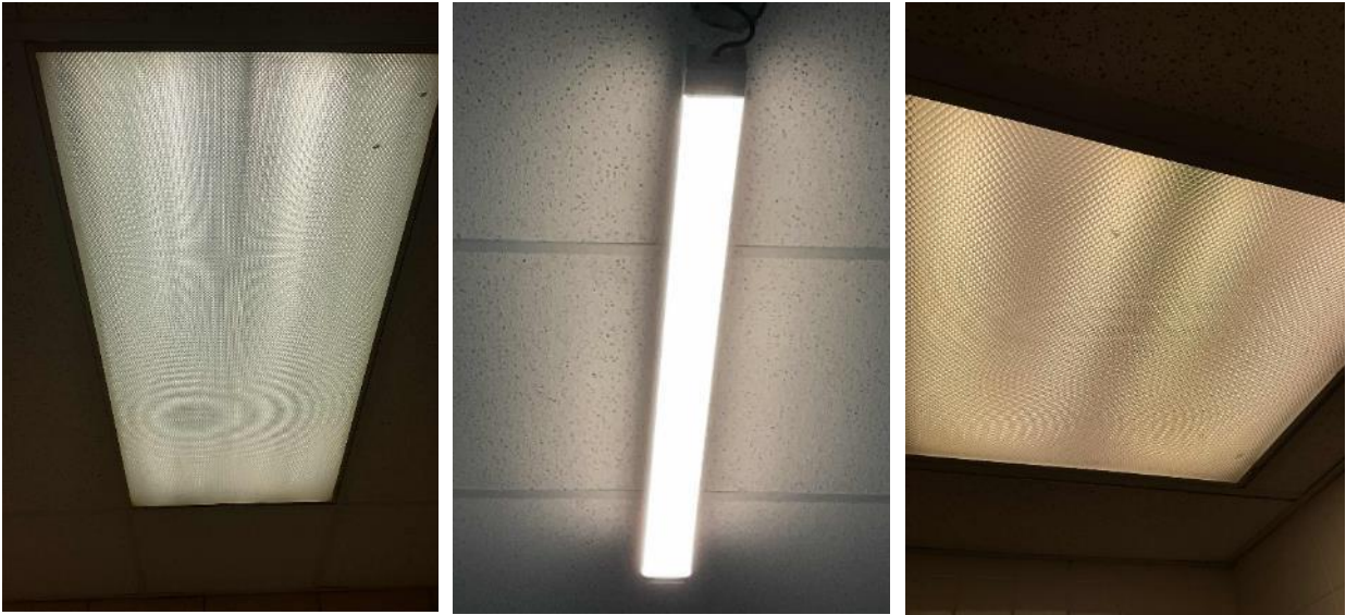
Linear Fluorescent T8 and LED Fixtures
