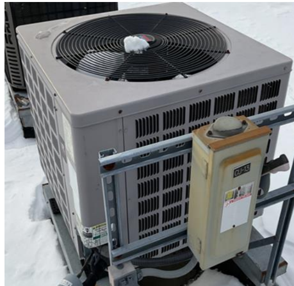
Thermal Zone Condensing Unit (CU)
