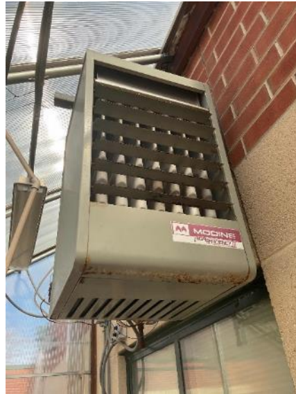
Typical Facility Unit Heater
