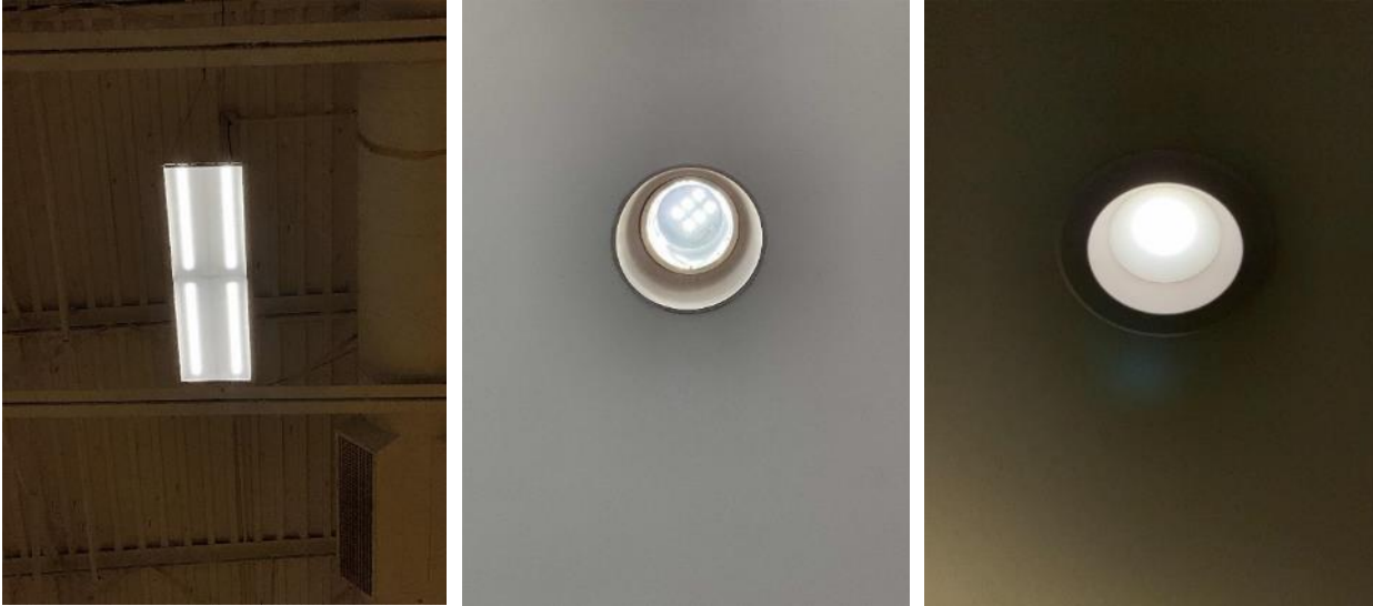
LED Fixtures in Gymnasium and Main Corridor
