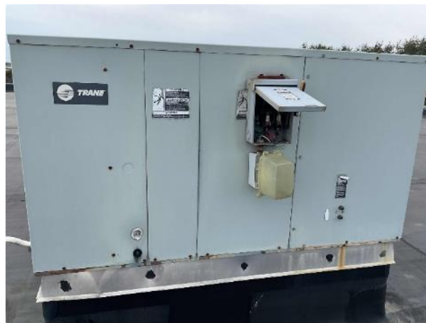
Trane RTU Mounted Above Classroom C-3
