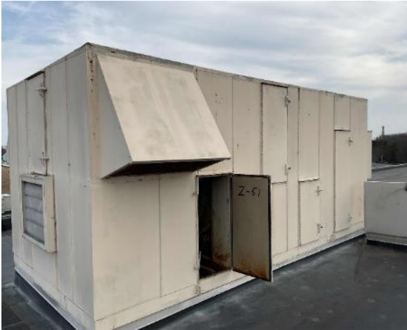
Heating Recovery Units
