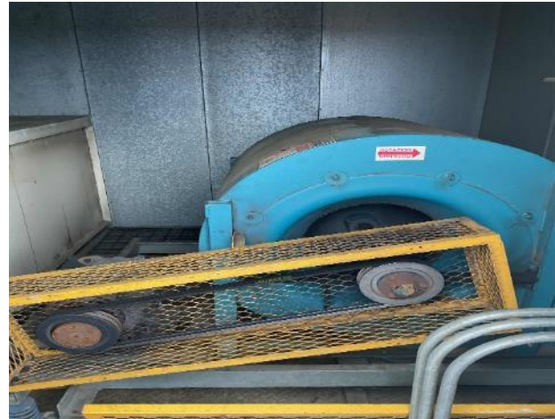
Heating Recovery Motors
