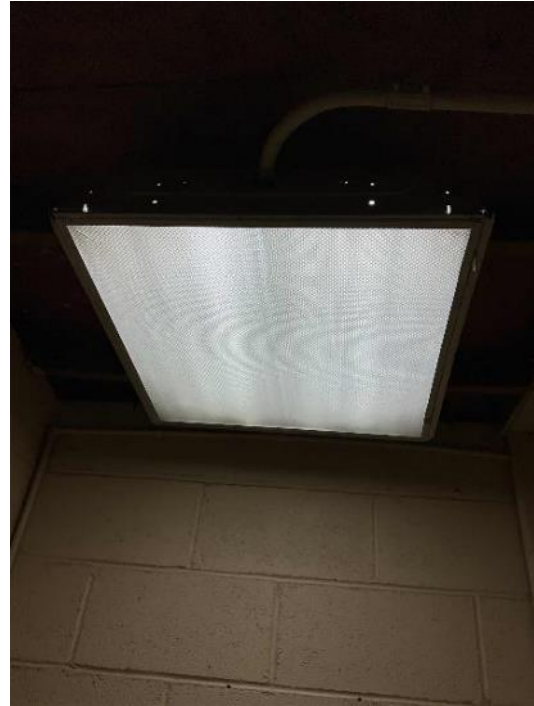
Fluorescent T8 U Bend Fixtures: Restroom
