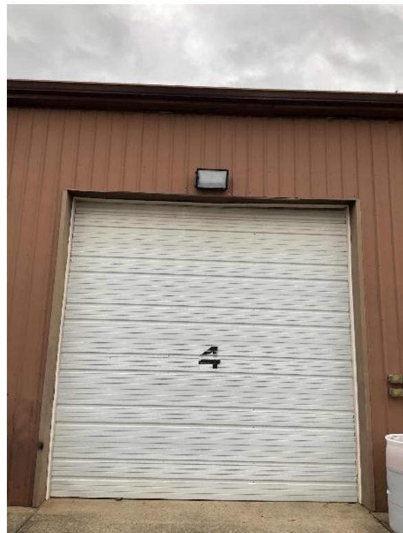
Building Overhead Doors
