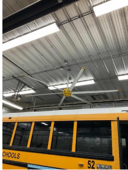
Destratification Fan: Garage
