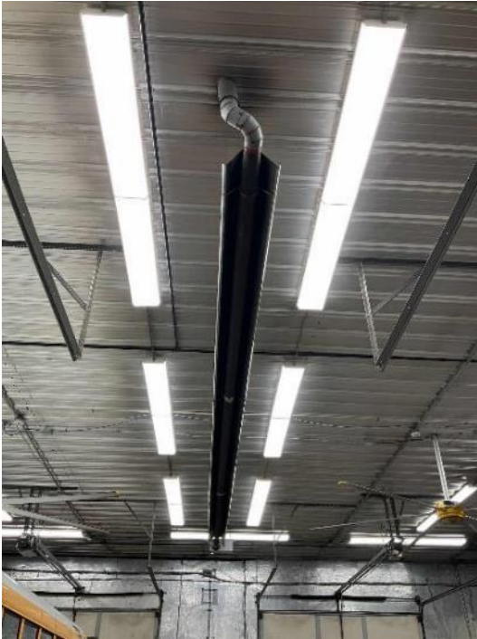
Fluorescent T8 Fixtures: Garage Area
