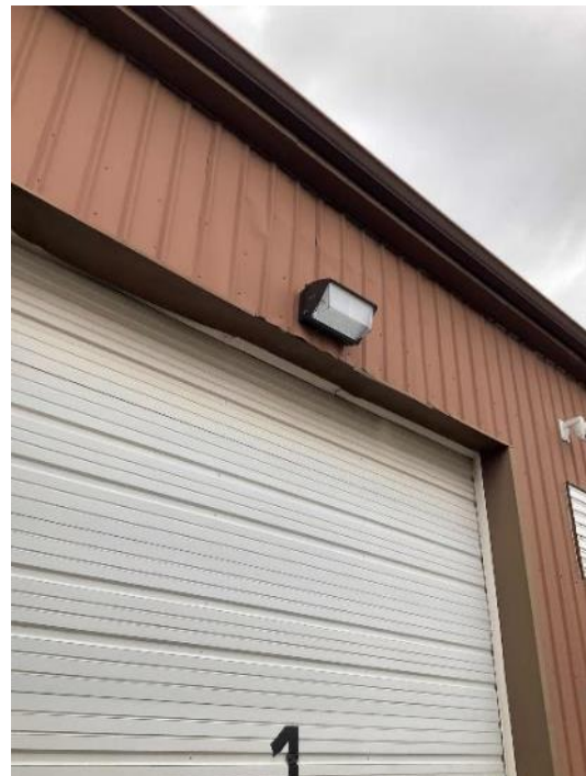
Exterior LED Fixtures
