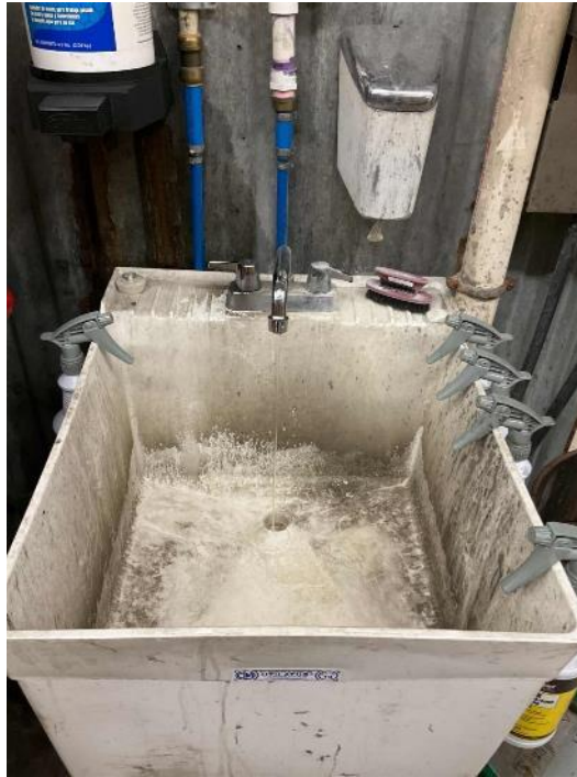
Garage Area Faucet
