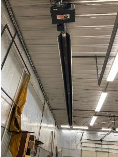
Infrared Heater - Garage Area
