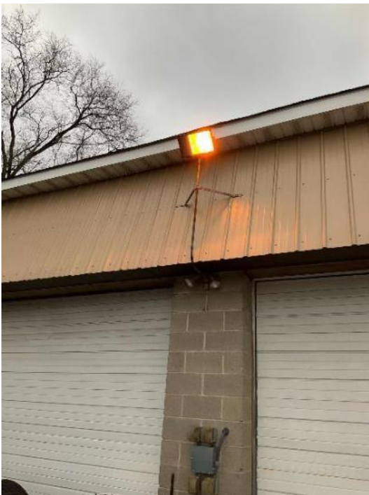
Exterior HID Fixtures
