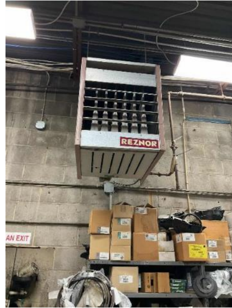
Forced Air Furnace-Garage
