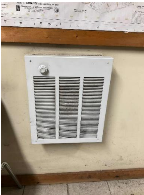
Electric Resistance Heater - Office
