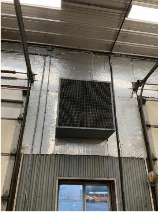
Exhaust Fan: Garage
