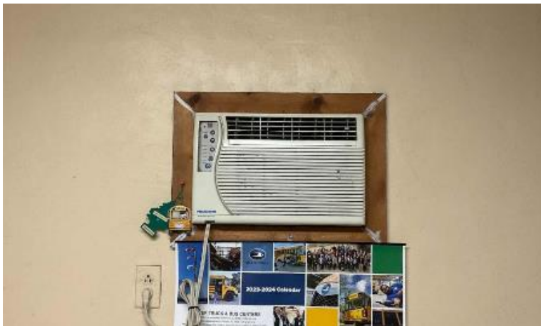
Office Area - Window Air Conditioner
