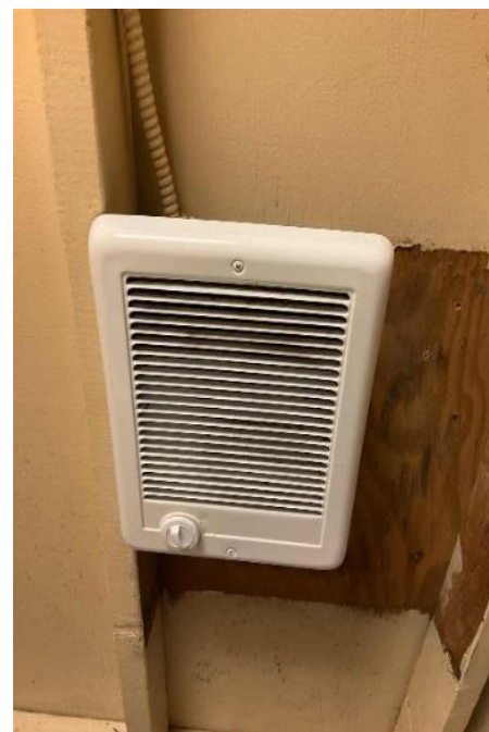
Electric Resistance Heater - Restroom
