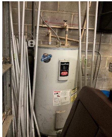
Domestic Hot Water Heater
