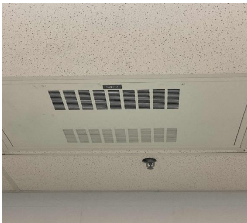
Ceiling-Mounted Unit Heater
