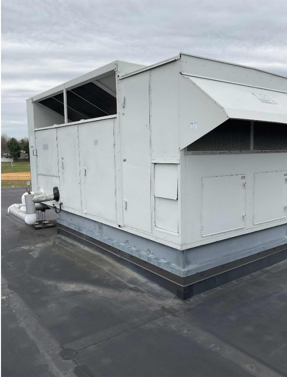
Typical RTU with Hot Water Heating
