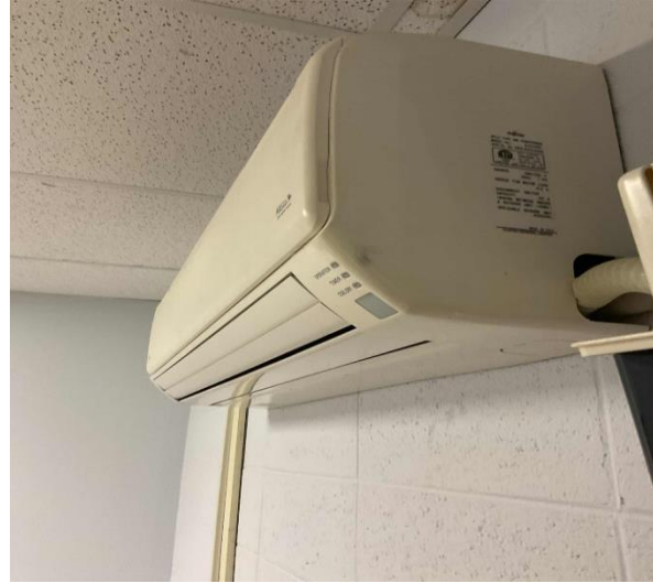
Fujitsu Air-Sourced Heat Pump Indoor Unit
