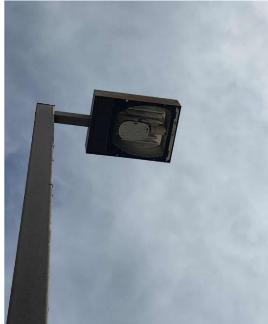
LED-Retrofit Street Lighting
