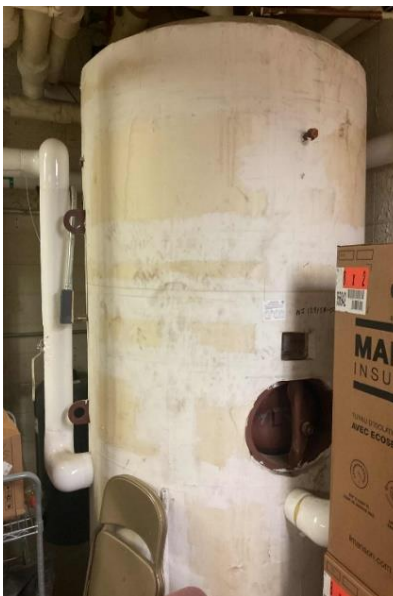
Domestic Hot Water Storage Tank
