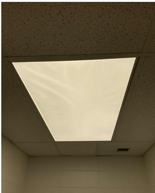
LED Light Panels in Restrooms
