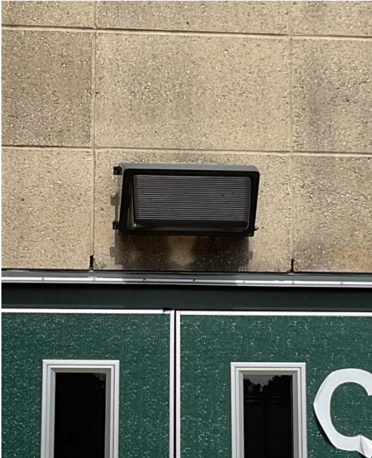
LED Wall Packs
