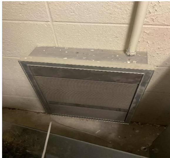
Mechanical Room Unit Heater
