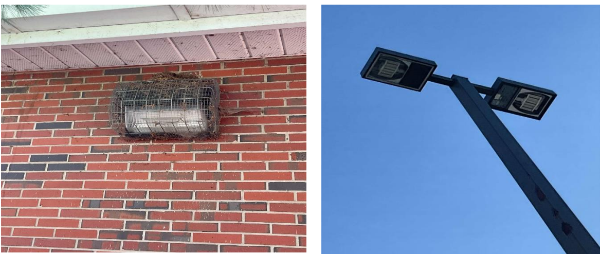
LED Parking Lot Lighting
