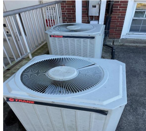
Typical Condensing Unit in Old Building
