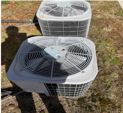
Typical Condensing Unit in New Building
