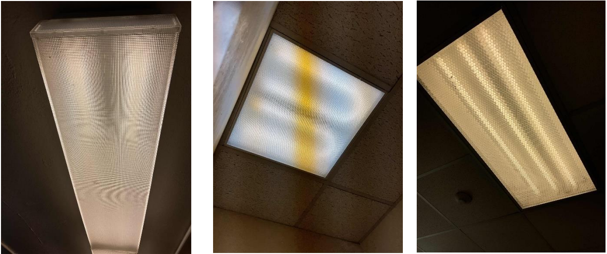
Typical Linear Fluorescent Fixtures Present in Both Buildings
