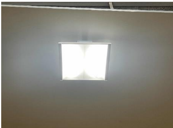
Typical LED Fixtures in Gymnasium
