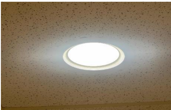
Typical LED Fixtures in Corridors
