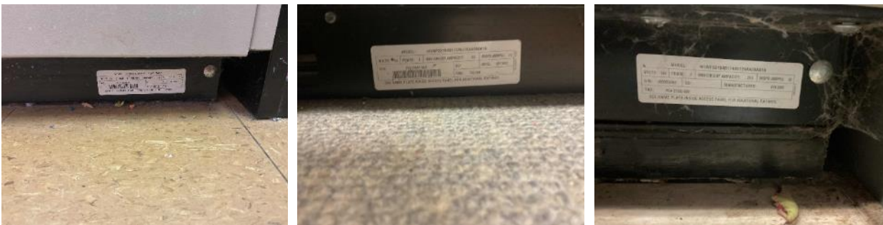
Typical Unit Ventilator Ages
