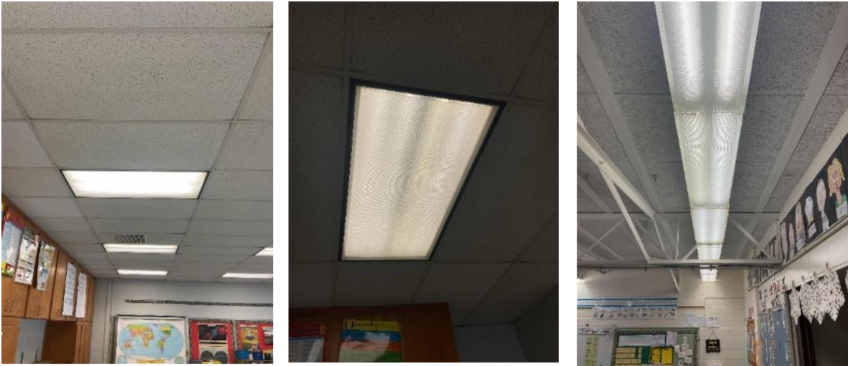
Typical T8 Linear Fluorescent Light Fixtures
