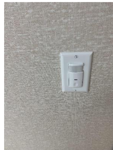
Occupancy Sensors in TCU
