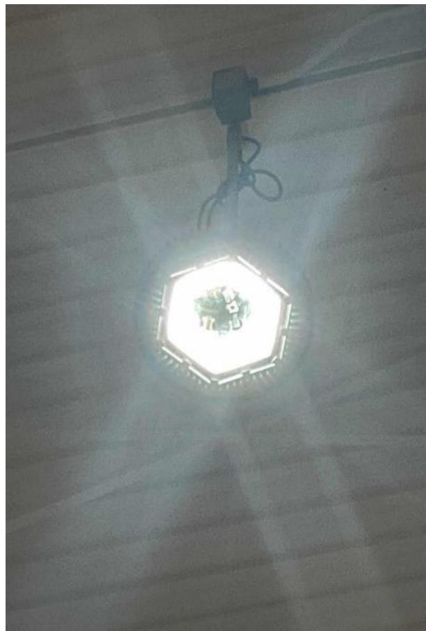
Typical LED Fixtures Multipurpose Room/Cafeteria
