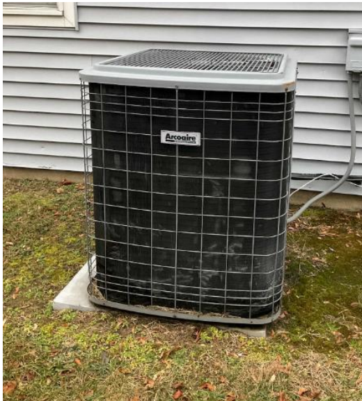
Split Air Source Heat Pump- Condensing Unit
