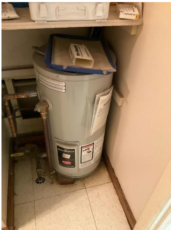
Electric Resistance Unit Heater
