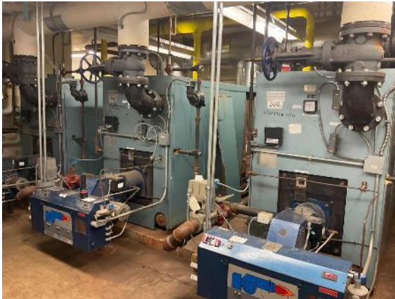
Hot Water Boiler
