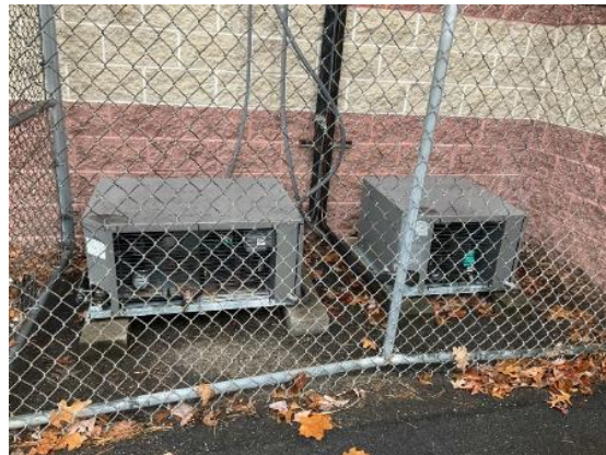
Condensing Unit Walk-in Cooler and Freezer
