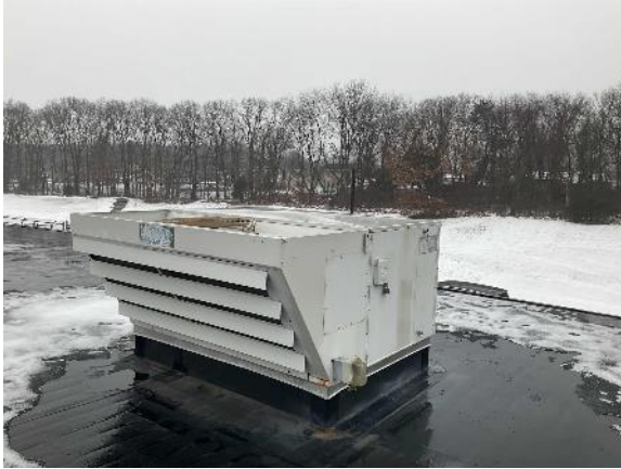
Package Unit-Faculty Room
