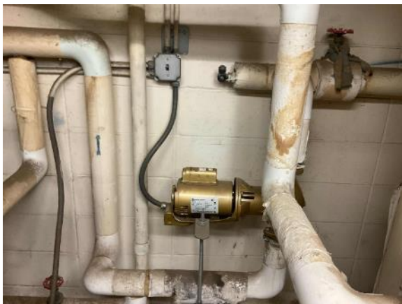
DHW Circulation Pump
