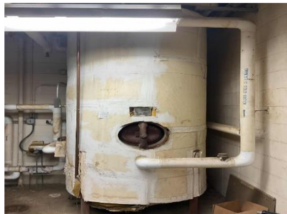
Domestic Hot Water Storage Tank
