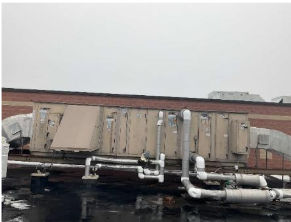
AHU-7 Block A and B
