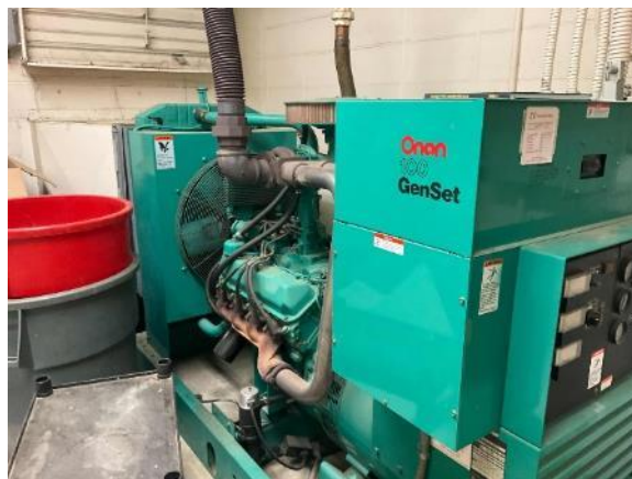
Natural Gas -Emergency Generator
