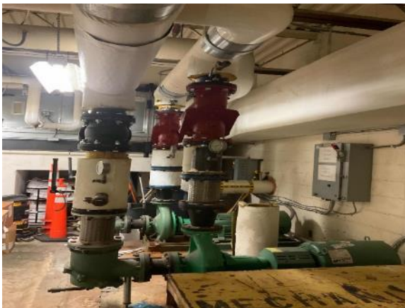
Old Hot Water Pump with VFD
