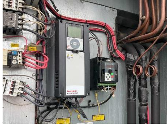
VFD-Supply and Return Fan (Gym Units)
