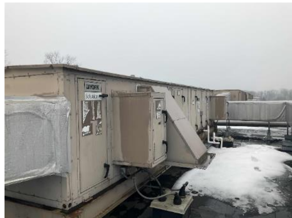
AHU-1 Block A Offices
