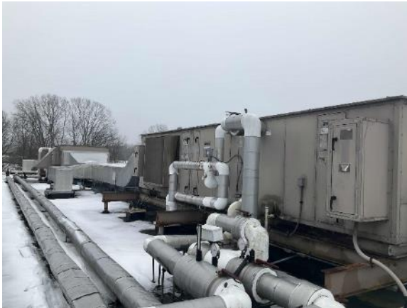
AHU 5-Block D
