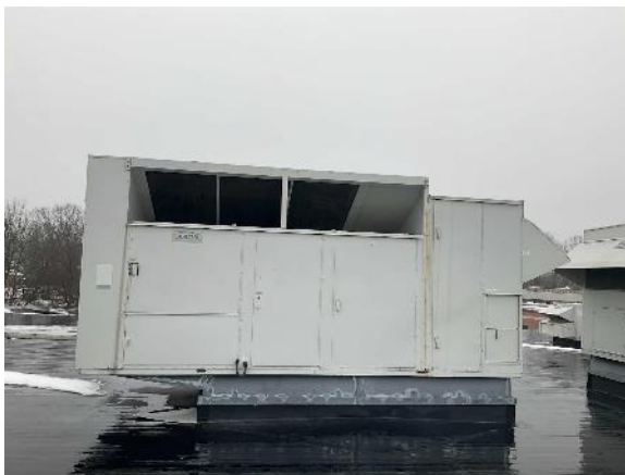
Package Unit-Gym Area
