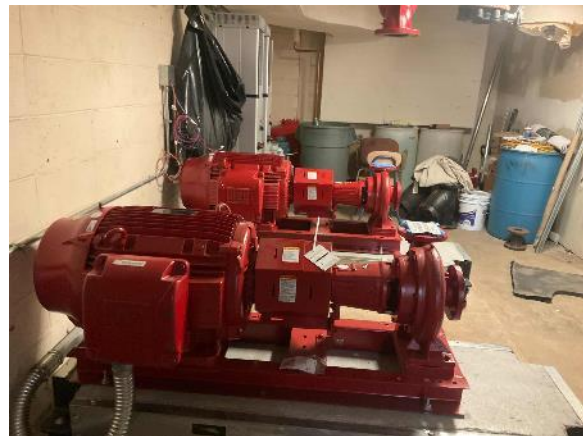
New Hot Water Pump with VFD
