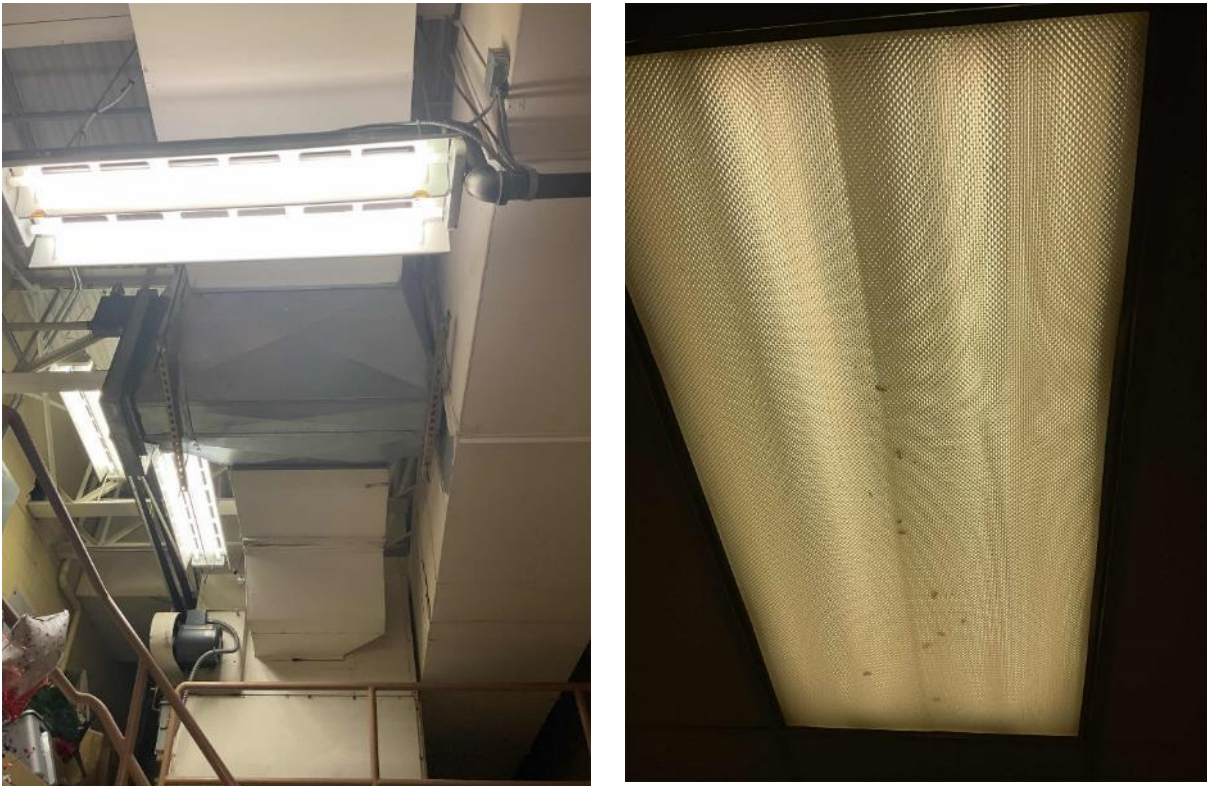
Typical T8 Linear Fluorescent Fixtures
