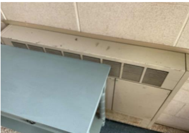
Typical Facility Unit Heater
