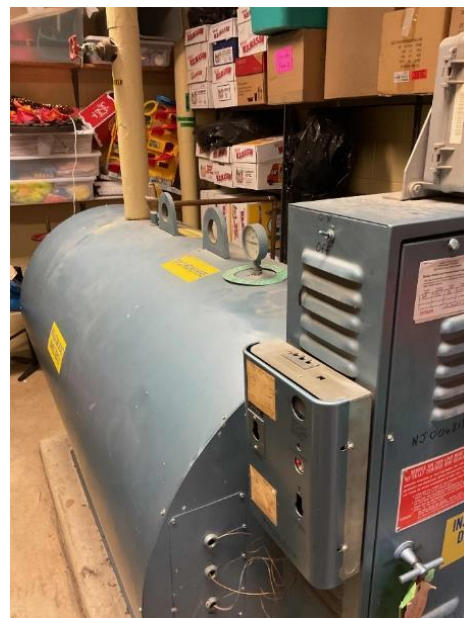
Electric Water Heater
