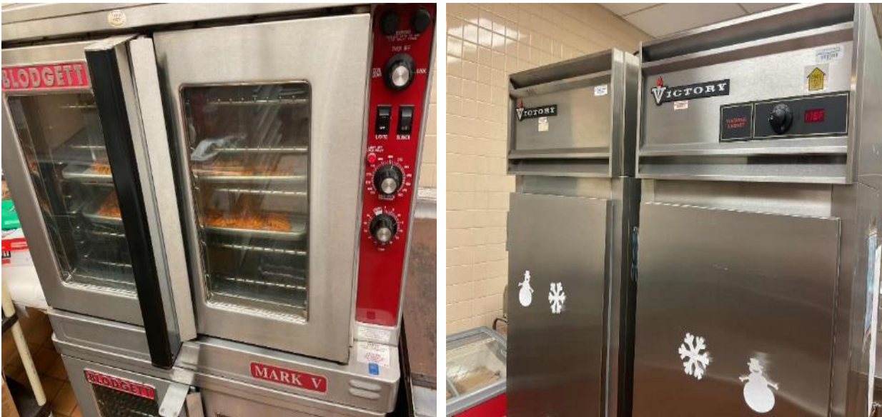
Typical Food Service Equipment
