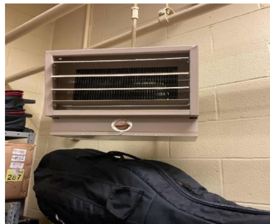
Stairwell Unit Heater
