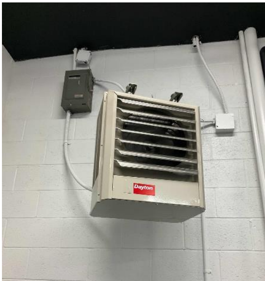
Electric Unit Heater-Pride Pavilion
