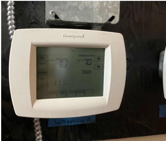
Thermostat- Unit Heater-O'Brien Hall
