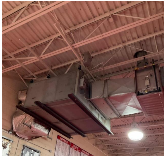
Make-Up Air Unit Heaters
