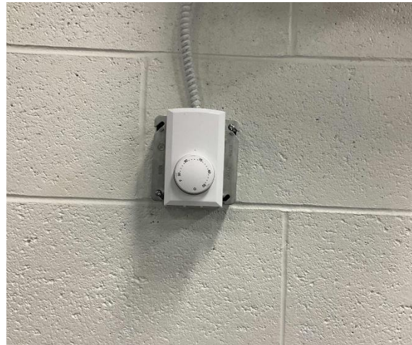
Thermostat- Unit Heater-Pride Pavilion
