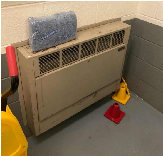
Electric Unit Heater
