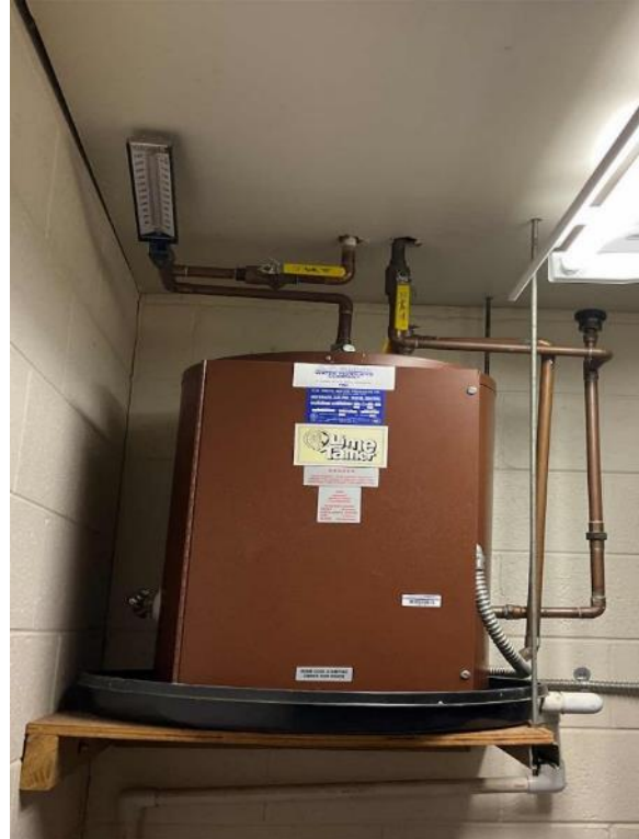
Electric Storage Water Heater-Snack Room
