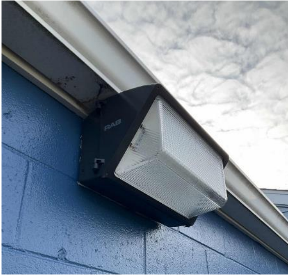
Exterior LED Fixtures
