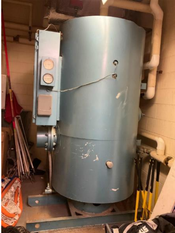
Electric Storage Water Heater-Locker Rooms
