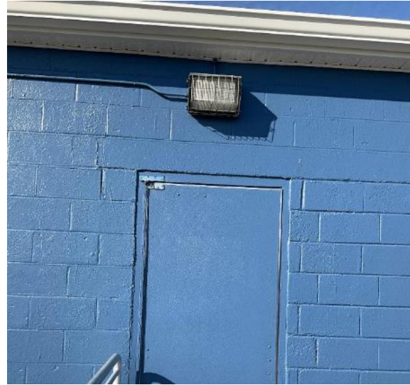
Exterior Metal Halide Fixtures
