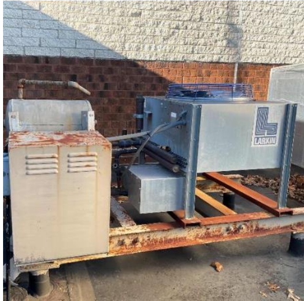
Dry Cooler- Office-9/10 Building
