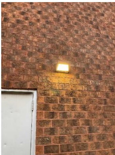
Exterior HID Wall Pack Fixtures
