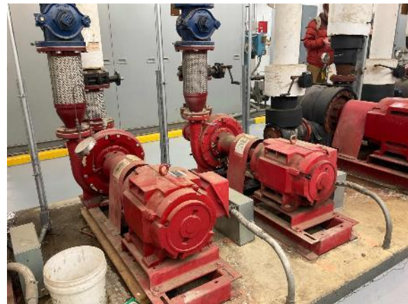
Heating Hot Water Pump-Core Building
