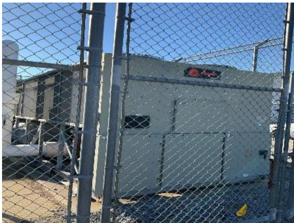
Air Cooled Chiller
