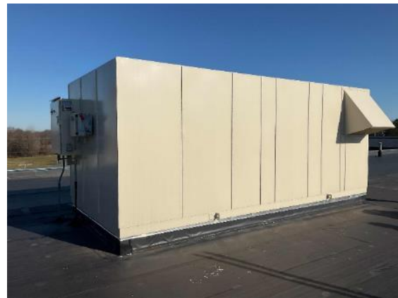
Heat Recovery Unit-Core Building
