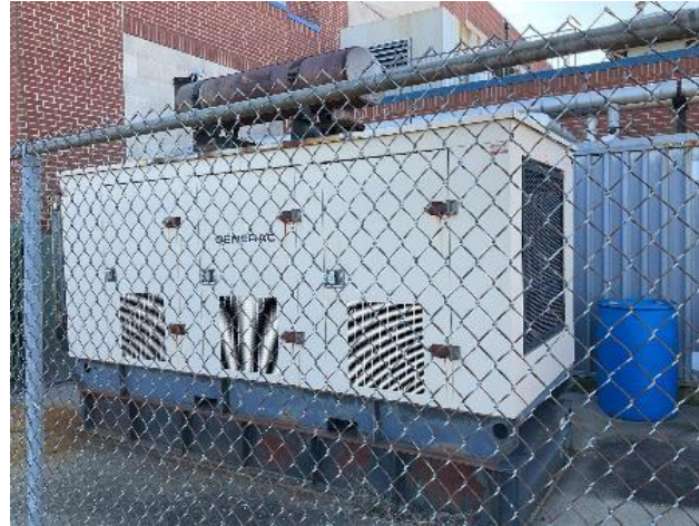
Diesel-Fired Emergency Generator
