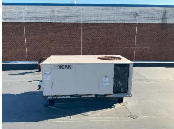
Package Unit-Kitchen Area
