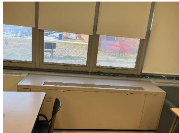
Typical Classroom Unit Ventilators
