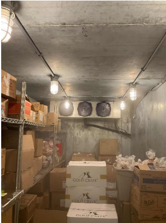
Low Temp Freezer: Kitchen 11/12 Building
