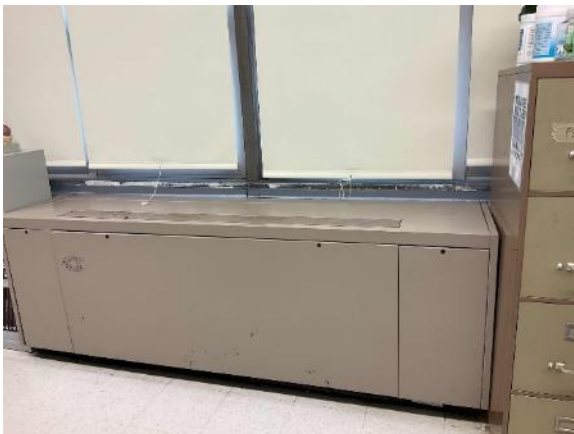
Typical Classroom Unit Ventilators
