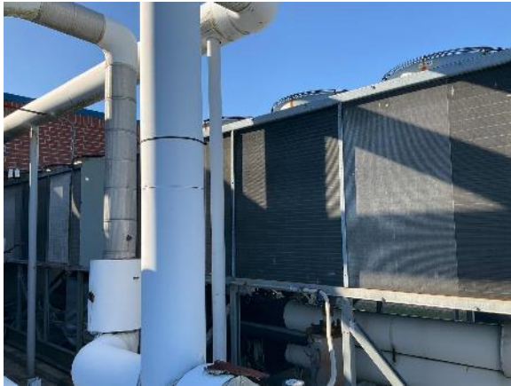
Air Cooled Chiller-Core Building
