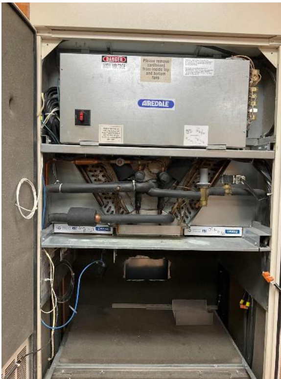
Package Heat Pumps-9/10 Building
