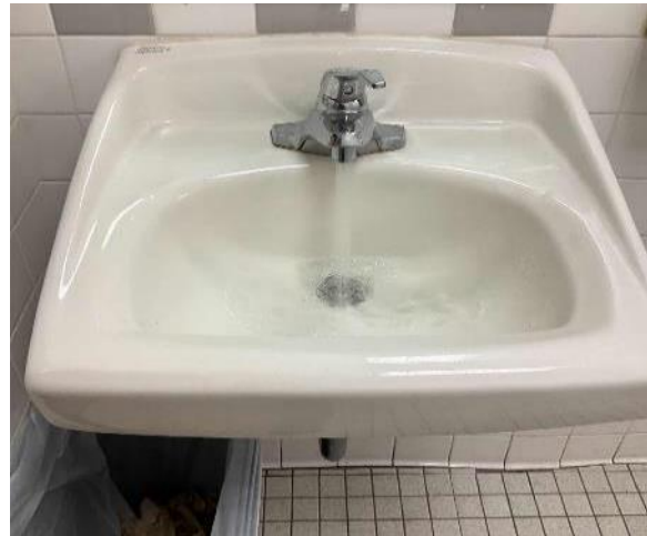
Typical Restroom Faucet-9/10 Building
