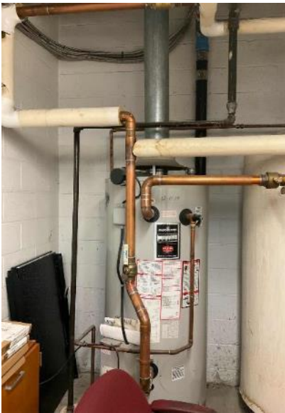
DHW Heater: Cafeteria-9/10
