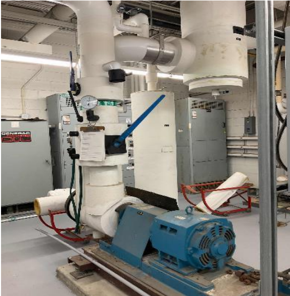
Chilled Water Pump
