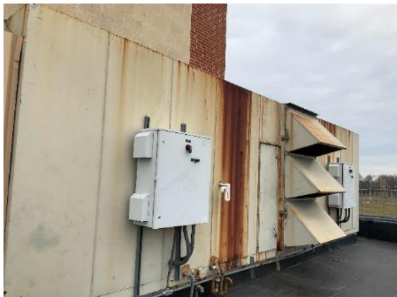
Air Handling Unit-9/10 Building
