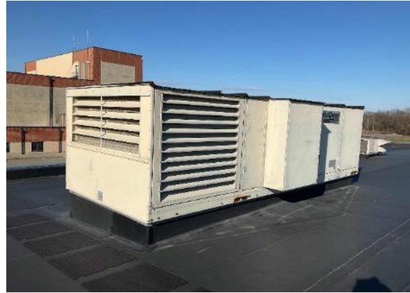
Air Handling Unit-Cafeteria (Core Building)
