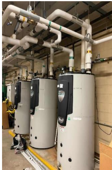
DHW Heater: Mechanical-9/10
