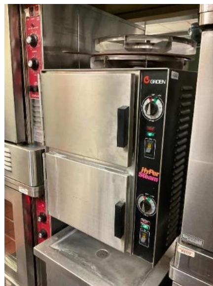
Electric Steamer-11/12 Building
