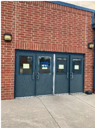
Exterior HID Wall Pack Fixtures
