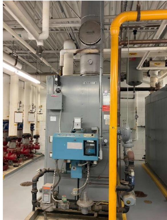
Hydronic Boiler-Core Building
