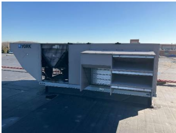
Package Unit-Gym Area-11/12
