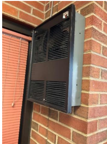
Unit Heater-Athletic Office-11/12
