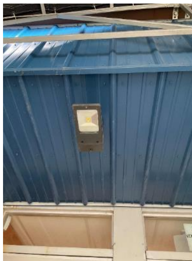
Exterior LED Fixtures
