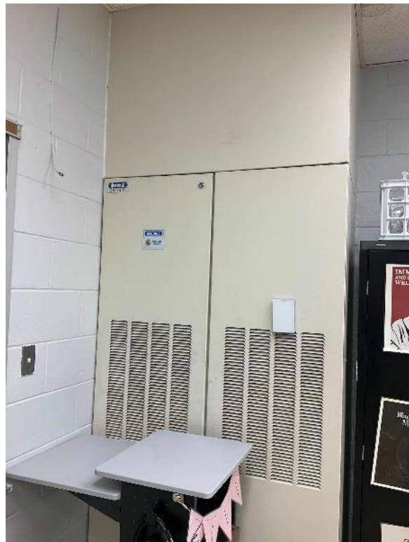
Package Heat Pumps-9/10 Building
