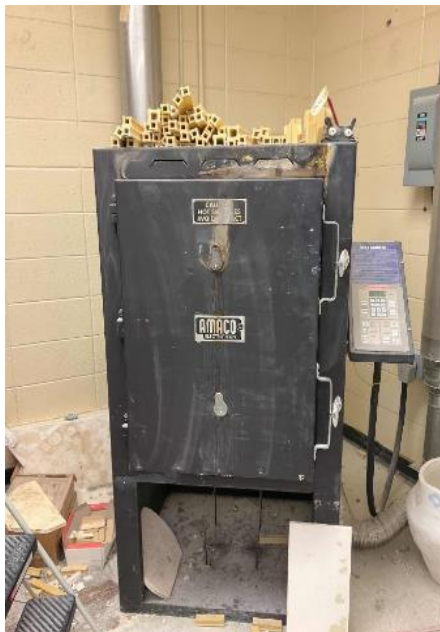
Typical Classroom Kiln
