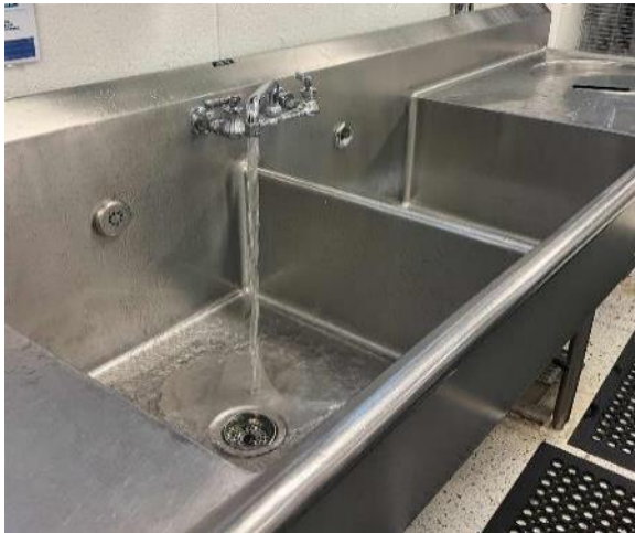
Typical Kitchen Faucet-9/10 Building
