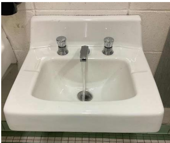
Typical Restroom Faucet-1/12 Building
