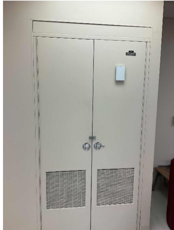
Package Heat Pumps-9/10 Building
