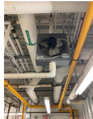
Unit Heater-Hot water-Mechanical Core room
