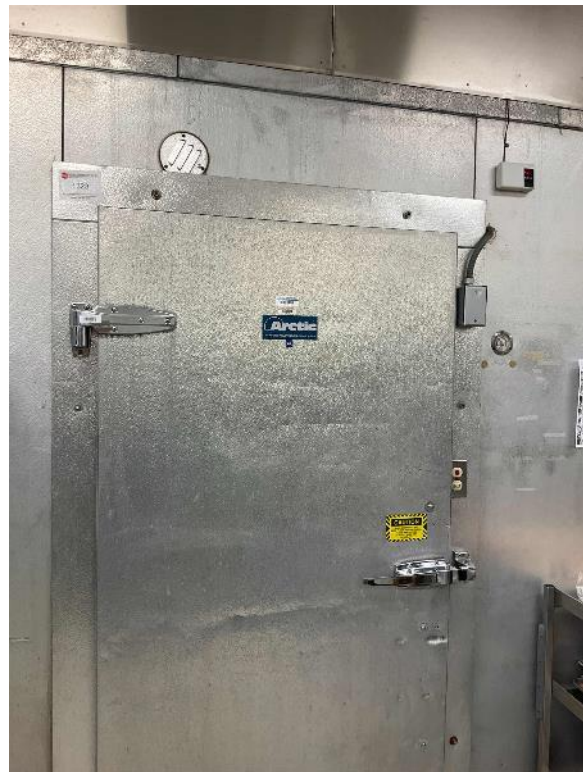
Medium Temp Freezer: Kitchen 9/10 Building
