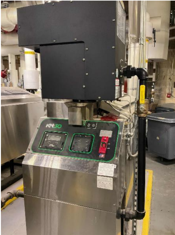
Condensing Boiler-11/12 Building
