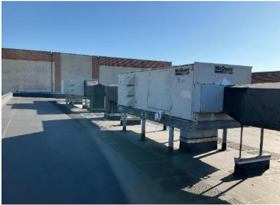
Air Handling Unit-Library (Core Building)
