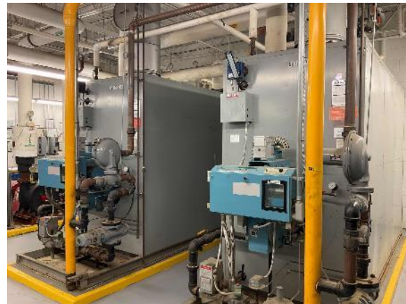
Hydronic Boiler-Core Building
