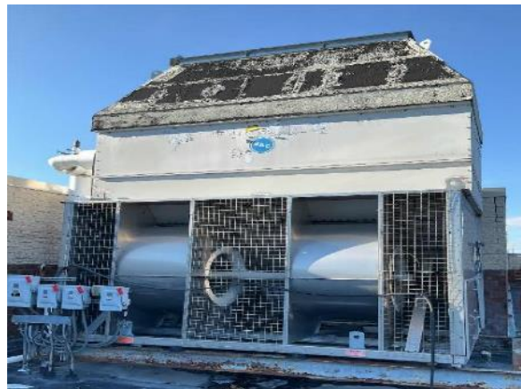
Cooling Tower-Water Source Heat Pump
