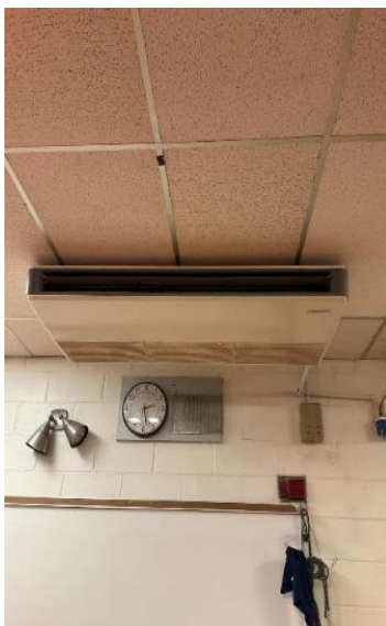
Indoor Unit- Split System-9/10 Building
