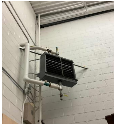
Unit Heater-Hot Water-Theatre
