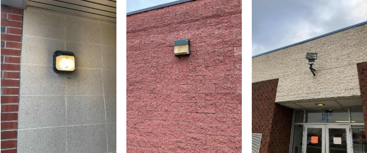
Exterior HID Fixtures
