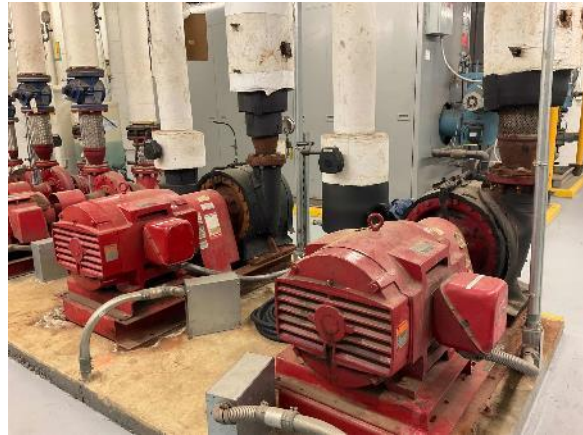
Chilled Water Pumps
