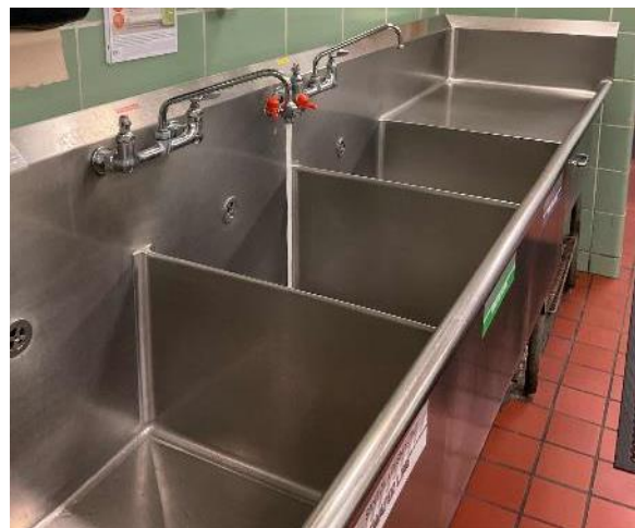
Typical Kitchen Faucet-11/12 Building
