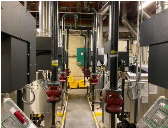
Condensing Boiler-11/12 Building
