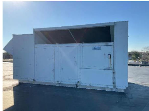
Package Unit-Gym Area-11/12
