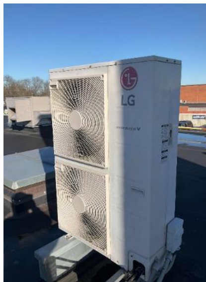
Split Air Source Heat Pump-11/12 Building
