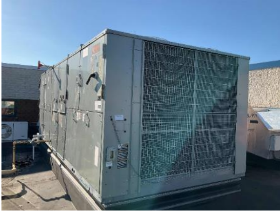
Package Unit with Gas Heat-Gym Area-9/10 Building
