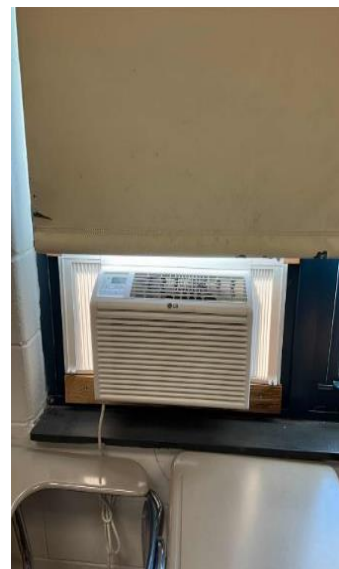
Window AC-9/10 Building
