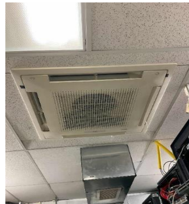
Ceiling Cassette- Split System-9/10 Building
