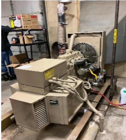
Gas Fired Emergency Generator
