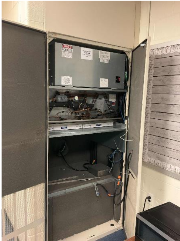
Package Heat Pumps-9/10 Building
