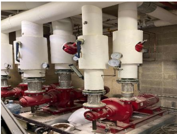
Heating Hot Water Pump-11/12 Building
