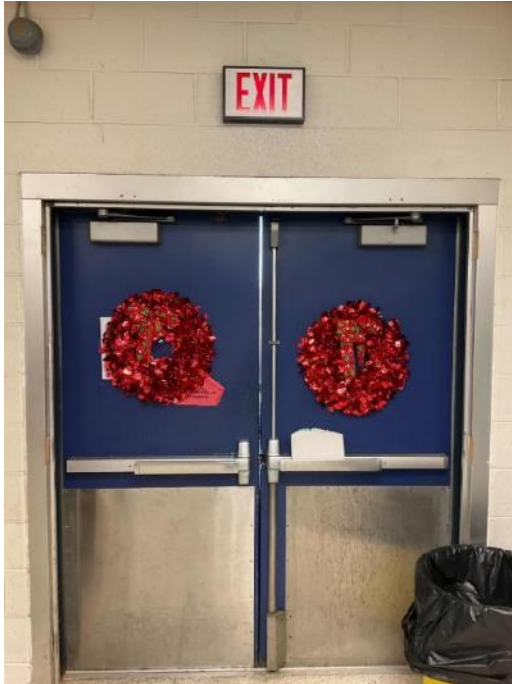
Door Gap: Infiltration-9/10
