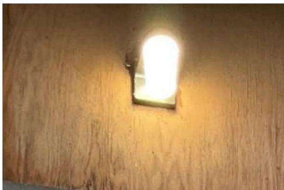
Exterior LED Fixtures
