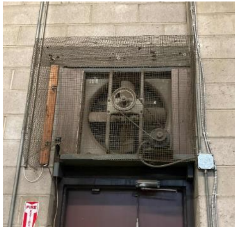
Exhaust Fan: Warehouse
