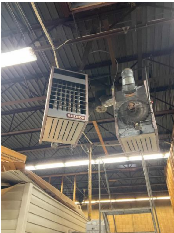
Forced Air Furnace: Warehouse
