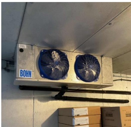
Walk-In Cooler: Evaporator
