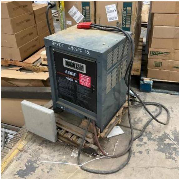
Forklift Battery Charger
