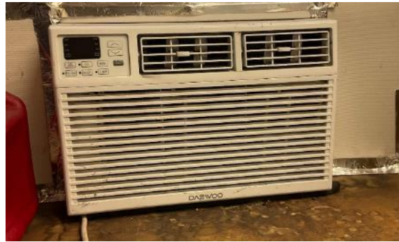
Office Area: Window Air Conditioner
