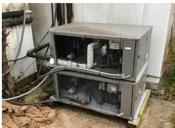
Low Temperature Freezer: Condensing Unit
