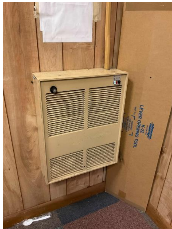
Unit Heater: Office
