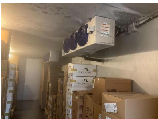
Walk-In Low Temperature Freezer: Evaporator
