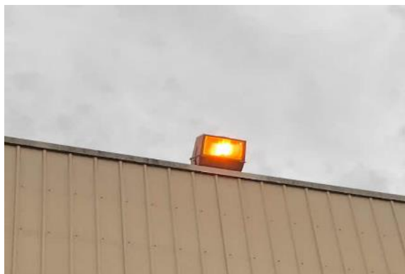
Exterior HID Fixtures
