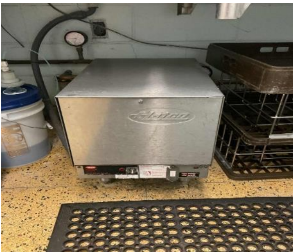
HATCO Booster Water Heater Attached to Dishwasher
