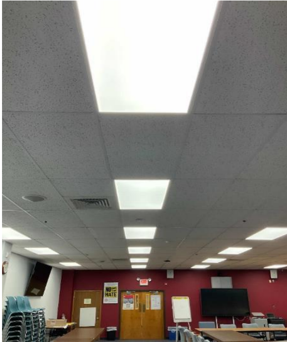
LED 2-foot x 4-foot Fixture-Conference Room
