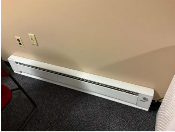
Electric Resistance Unit Heater
