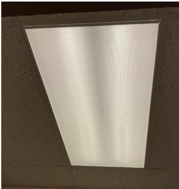
T8 Fluorescent Lamps
