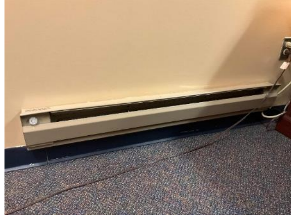
Electric Resistance Unit Heater
