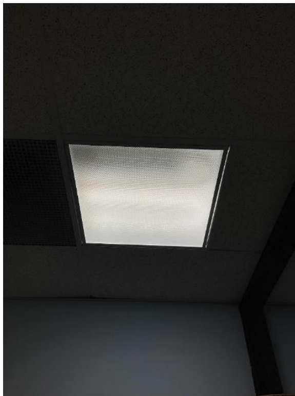
T8 Fluorescent U-Bend Fixture
