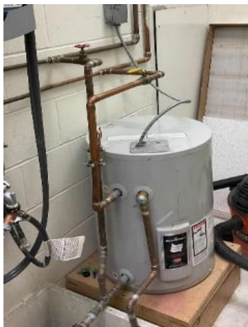
Domestic Hot Water Heater
