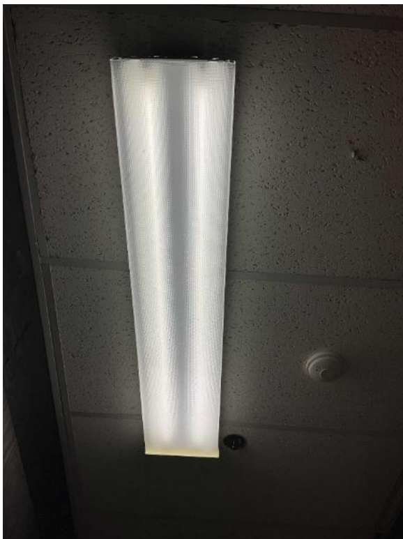
T8 Fluorescent fixture
