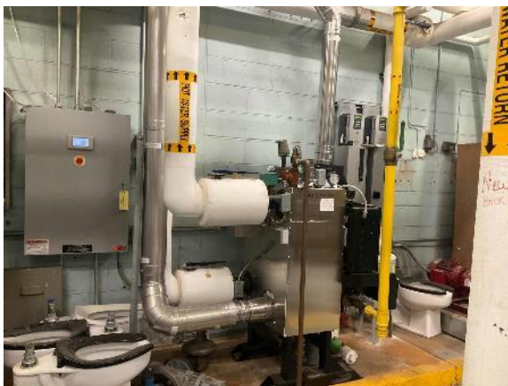
Hydronic Boiler New Building
