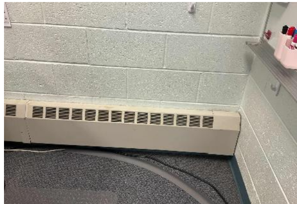
Hot Water Unit Heater
