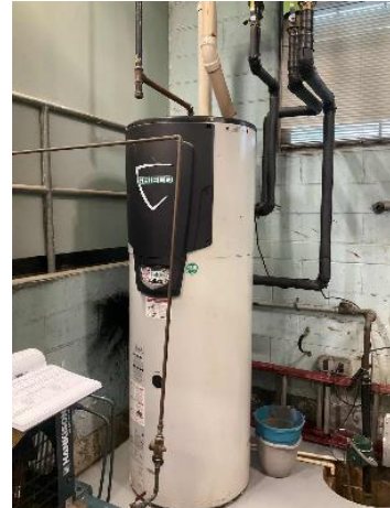
DHW Heater-Mechanical Room
