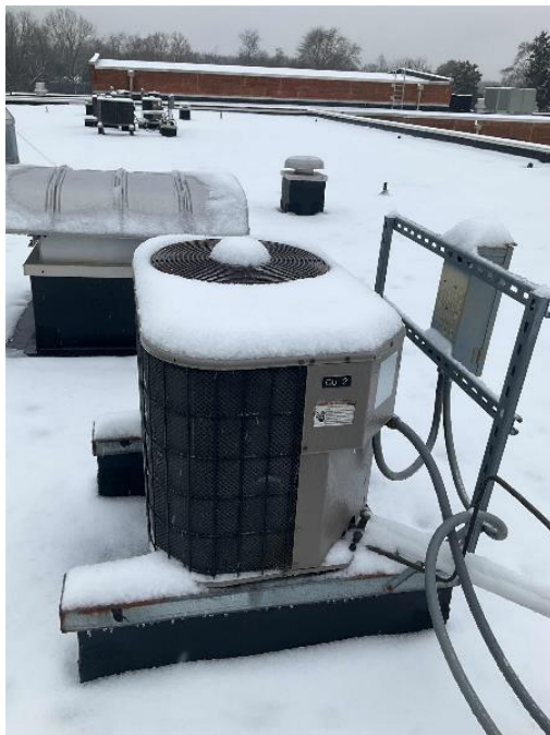
Condensing Unit- Unit Ventilator
