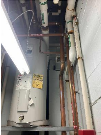
DHW Heater-Electrical Room
