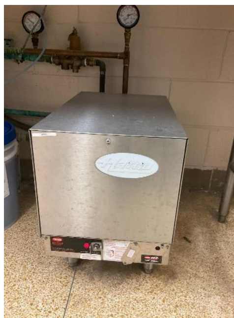
Booster Heater- Dishwasher
