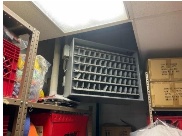
Hot Water Unit Heater
