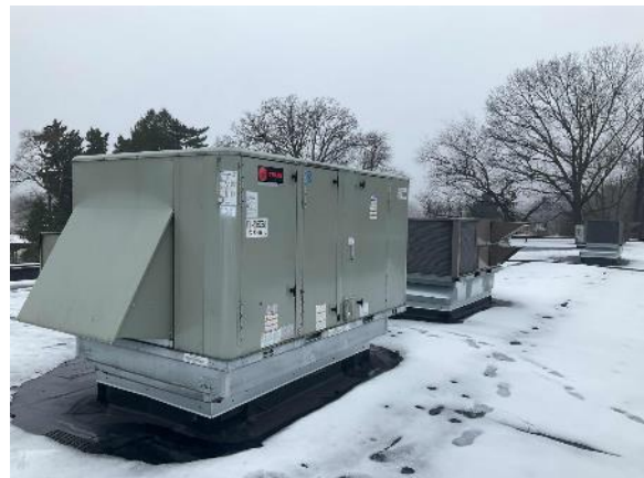
Rooftop Packaged Unit-Gym Area
