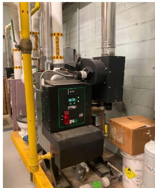
Hydronic Boiler-New Building
