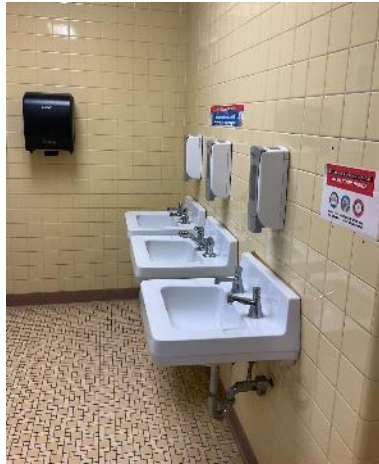
Typical Restroom Sinks
