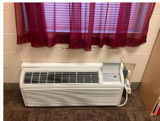
Through the wall Air Conditioning Unit
