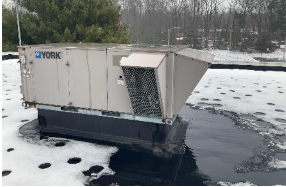
Rooftop Packaged Unit-Cafeteria
