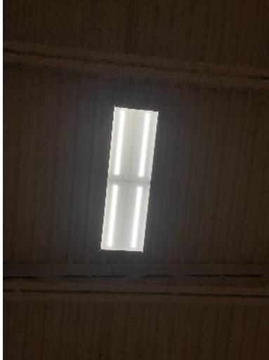
LED Fixture- Gymnasium
