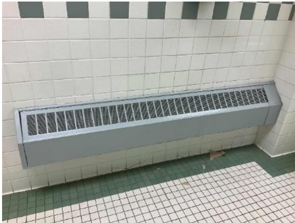
Unit Heater- Locker Room
