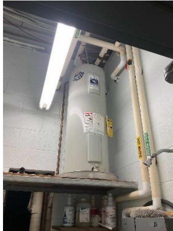
DHW Heater-Storage Room
