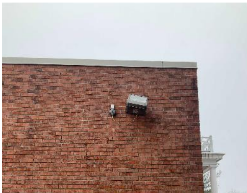
Exterior HID Fixture
