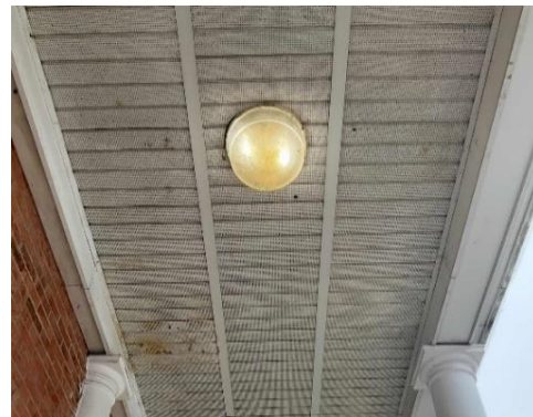
Exterior LED Lamps
