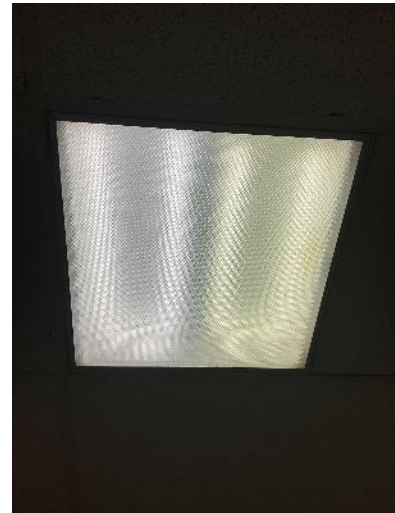
Fluorescent Fixtures- Corridor
