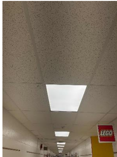
LED Fixture 2 x 4 - Corridor
