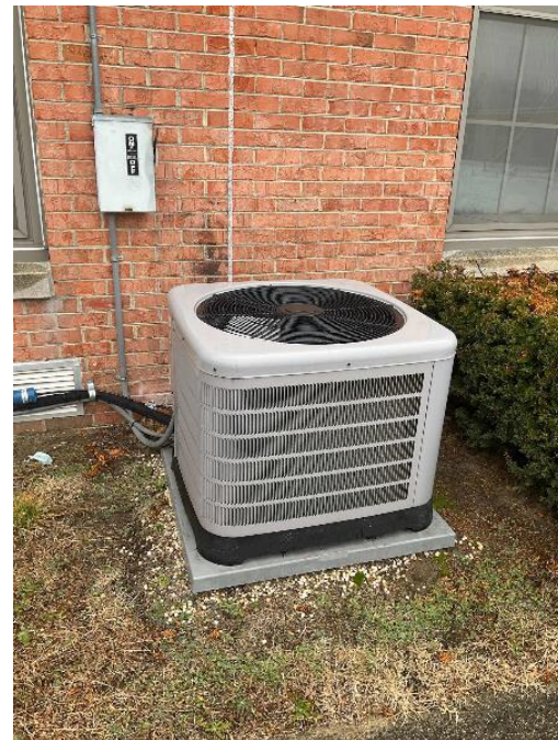
Condensing Unit- Unit Ventilator
