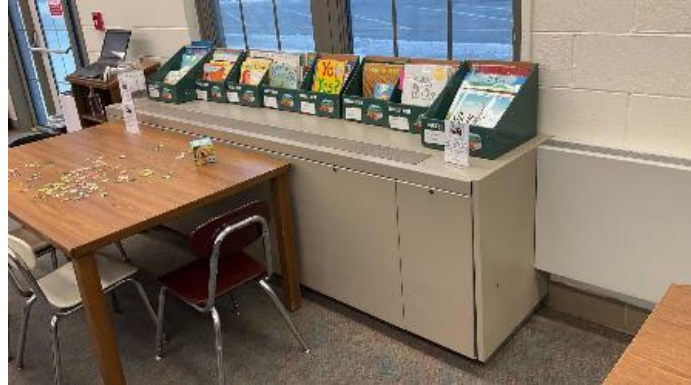
Typical Classroom Unit Ventilator
