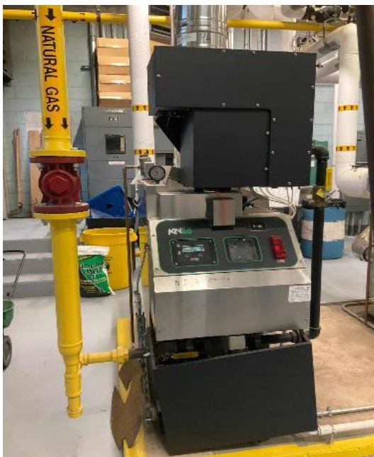
Hydronic Boiler-Original Building
