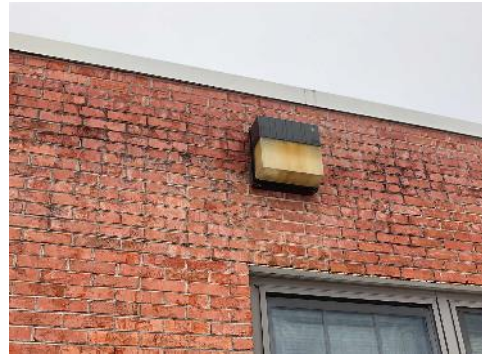
Exterior Metal Halide Wall Pack Fixtures
