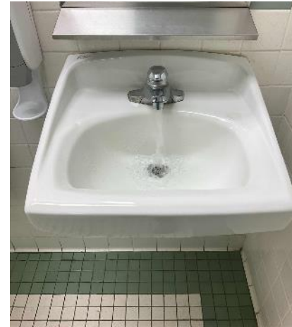
Typical Restroom Sinks
