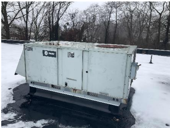
Rooftop Packaged Unit-Hallway
