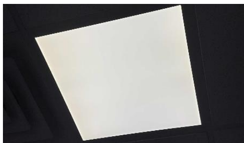
LED 2-foot x 2-foot Fixture
