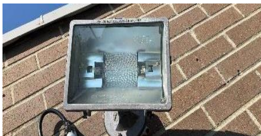
Exterior HID Fixture
