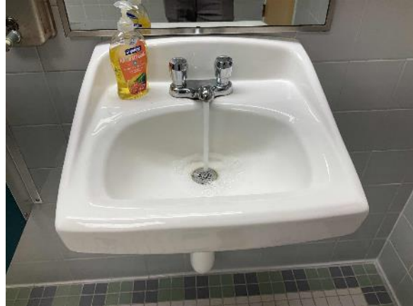
Typical Restroom Faucet
