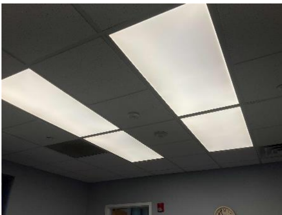
LED 2-foot x 4-foot Fixture
