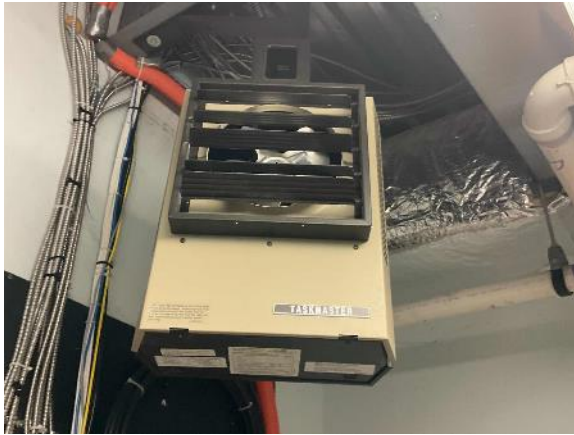
Electric Resistance Heater- Mechanical Room
