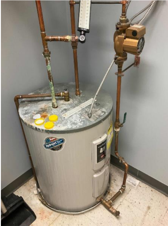
Electric Storage Tank Water Heater
