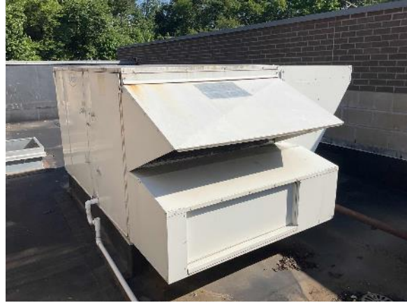
Packaged Rooftop Unit
