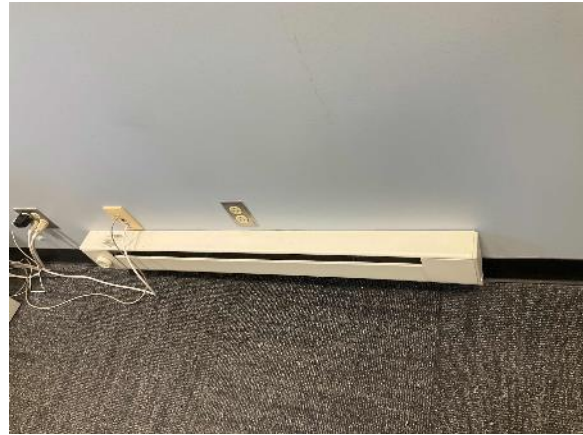
Electric Resistance Heater- Offices
