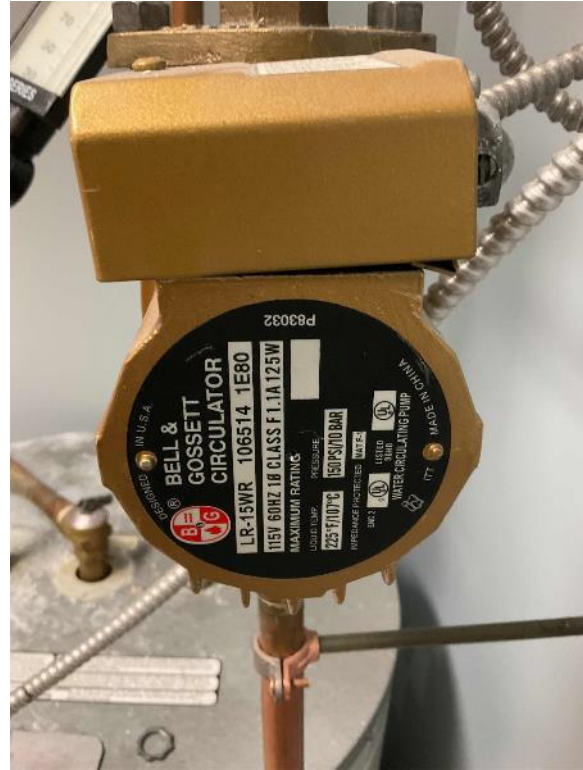
DHW Circulation Pump
