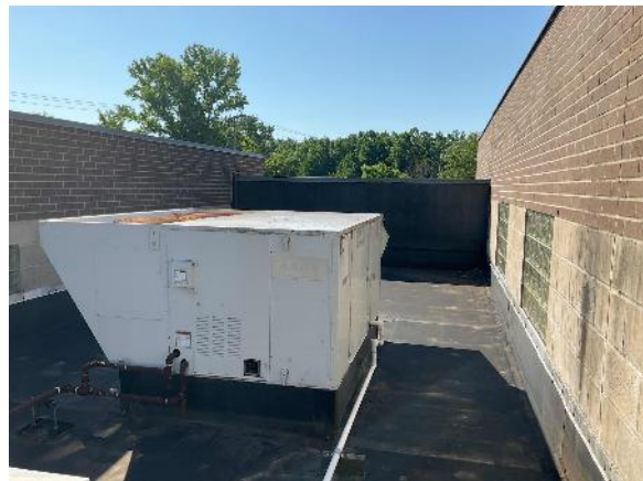
Packaged Rooftop Unit
