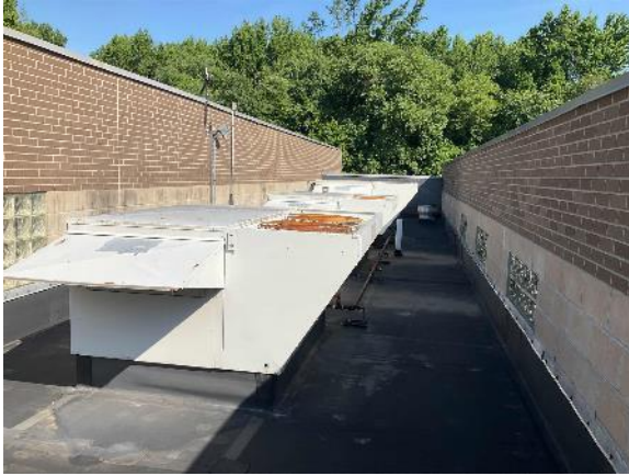
Packaged Rooftop Units
