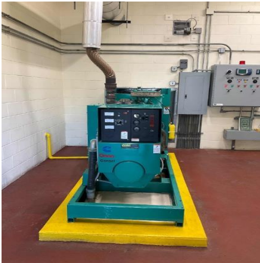
Natural Gas Standby Generator at Elizabeth Hills
