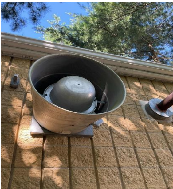
Exhaust Fan at Elizabeth Hills
