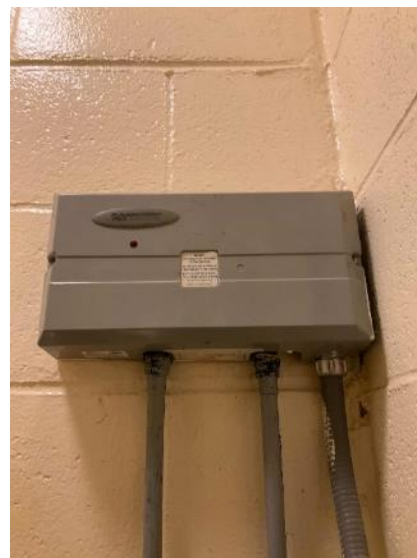
Tankless Heater at Hawkins
