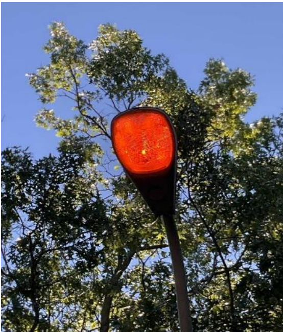
High Pressure Sodium Cobrahead with failed photocell (Elizabeth Hills)
