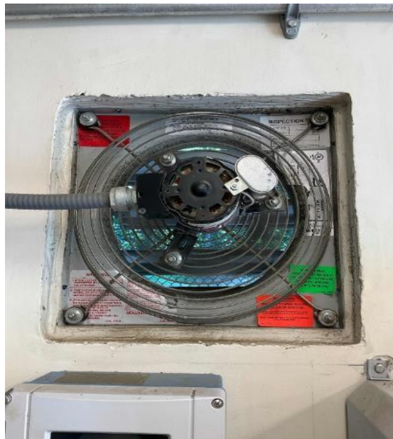
Exhaust Fan at Texas Road
