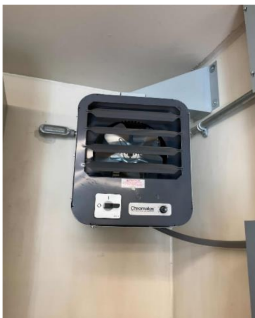
5 kW Unit Heater at Texas Road
