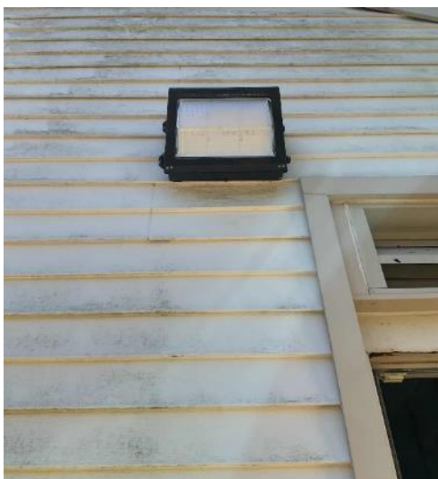
LED Wall Pack at Conover Hills
