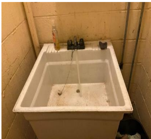
Sink at Hawkins
