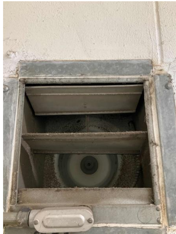
Exhaust Fan at Conover Hills
