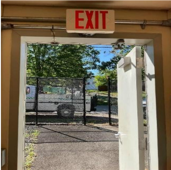
LED Exit Sign at Texas Road
