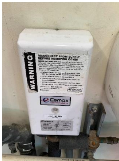
Tankless Heater at Greenwood Road
