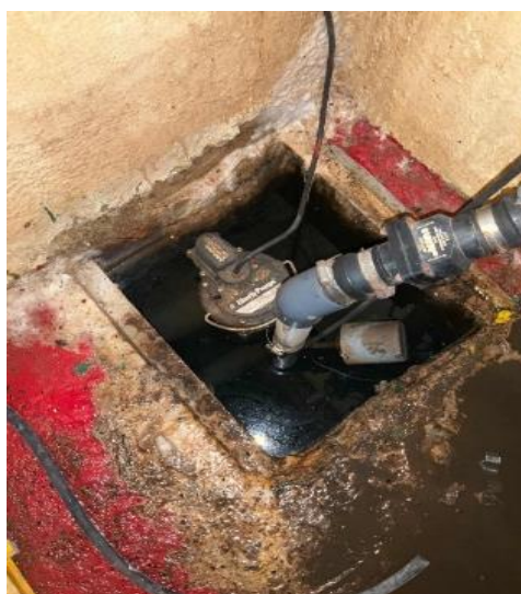
Sump Pump at Hawkins
