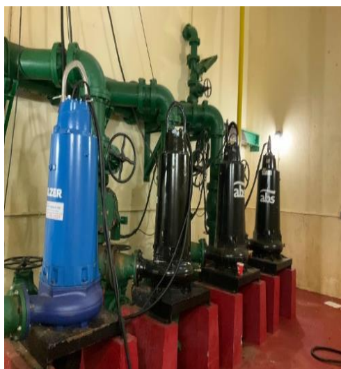
Sewage Pumps at Hawkins
