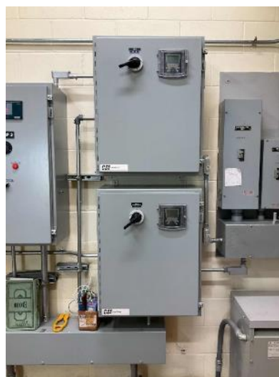
Sewage Pump VFDs at Elizabeth Hills
