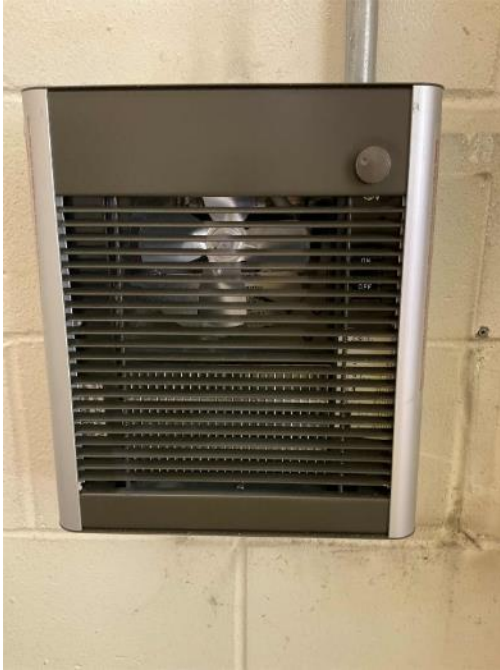
2 kW Unit Heater at Conover Hills
