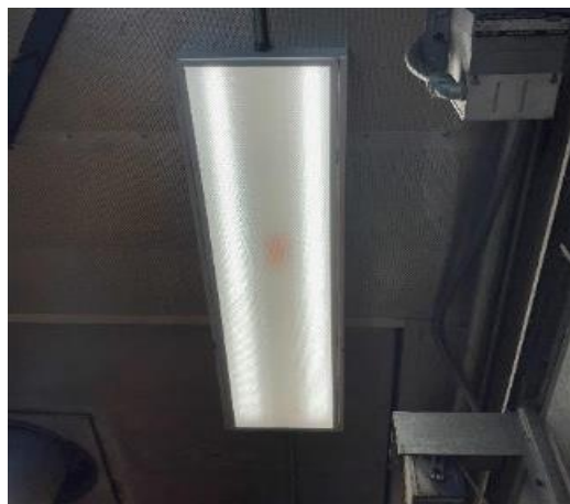
Fixture retrofitted with LED Tubes at Hawkins
