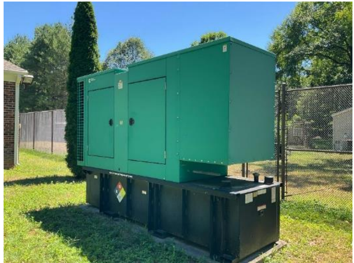
Diesel Standby Generator at Hawkins
