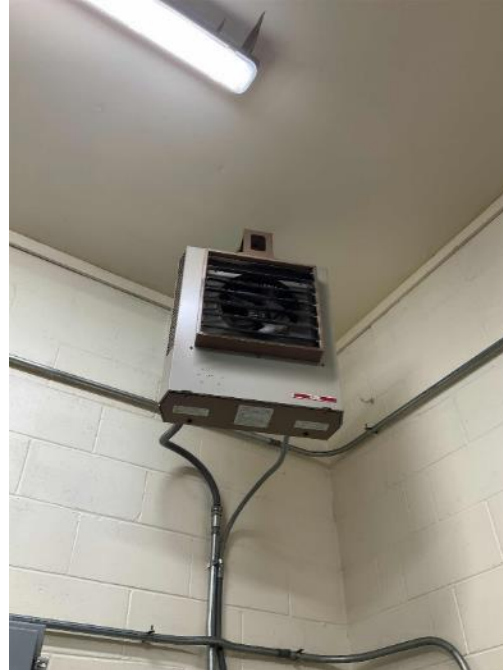
7.5 kW Unit Heater at Elizabeth Hills
