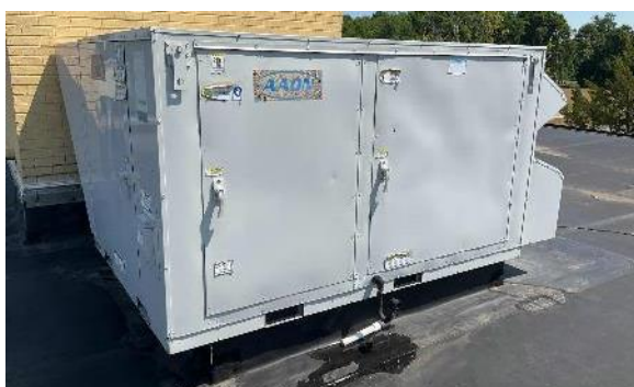
Rooftop Package Unit: FMB
