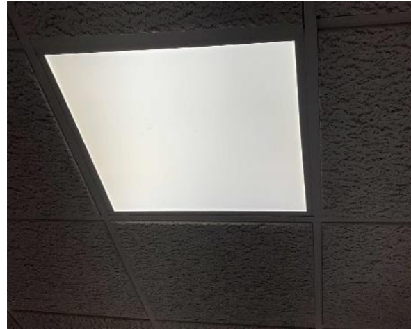
LED 2-foot Xx2-foot Fixture: Old Admin Building
