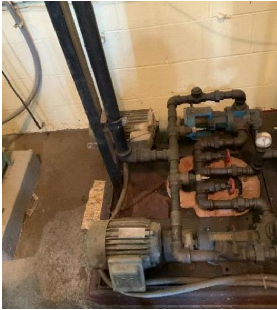
Boiler Feed Water Pump: FMB
