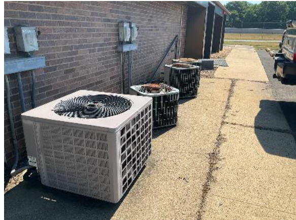
Split Condensing Unit: Old Admin Building
