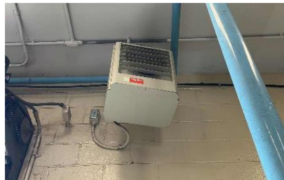
Electric Resistance Heater: Nitrification Building
