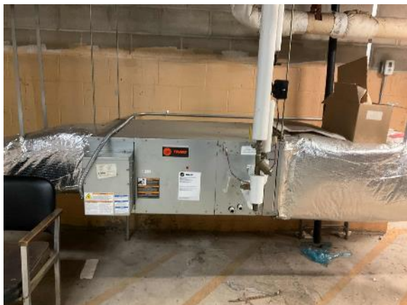
Air Handling Unit: FMB
