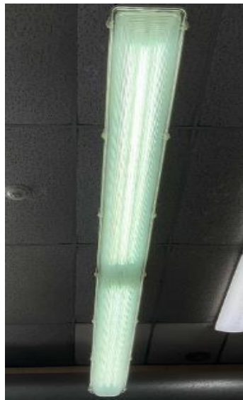
Linear T5 Lamps: Plant Maintenance Garage
