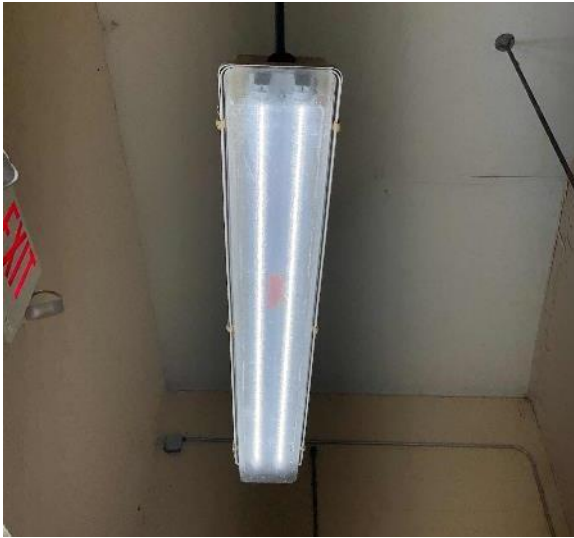
LED Linear Strip: Pump Station Control
