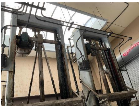
Debris Collection Motor (Bar Screen)
