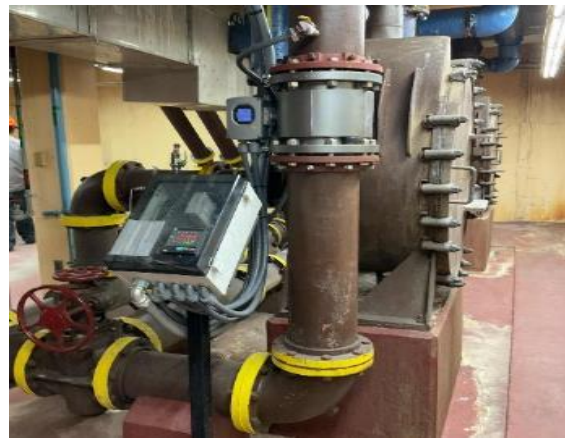
Heat Exchanger: Digester Building
