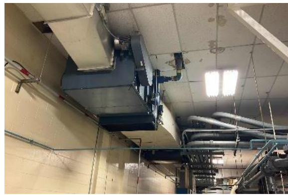
Air Handling Unit: Filter Building
