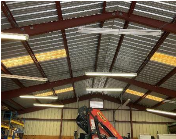
T12 Linear Fluorescent: Plant Storage
