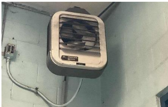
Electric Resistance Heater: Nitrification Building
