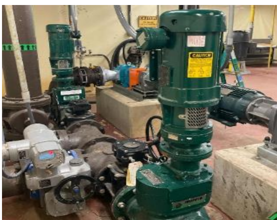
Raw Sludge Pump
