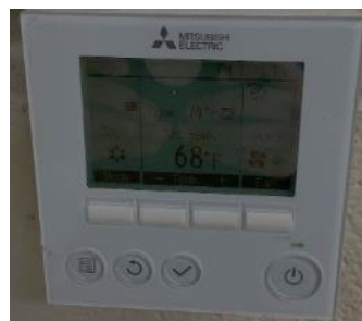
Thermostat: Pump Station Control
