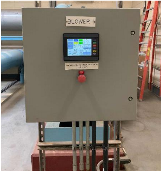
Aeration Blower 1: Control Panel
