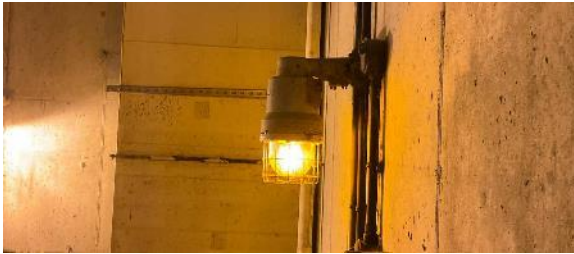
Incandescent Lamp: Pump Station Basement
