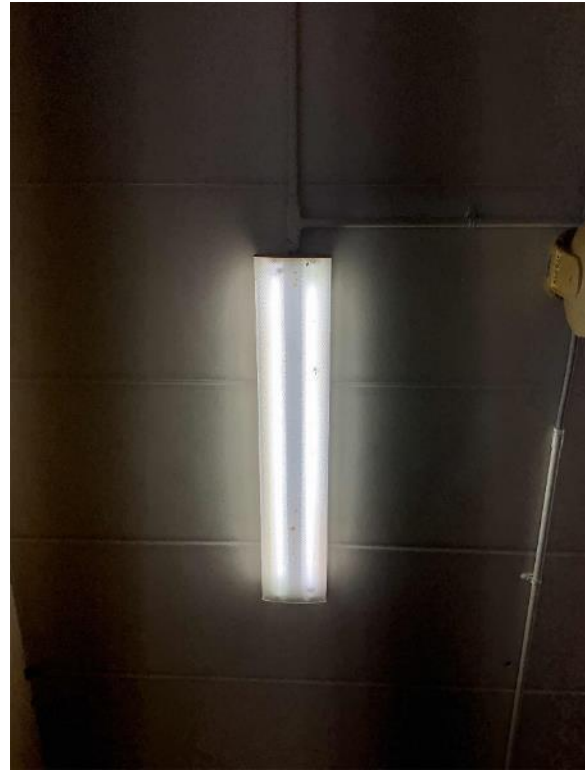
T8 Linear Fluorescent – U.V. Disinfection
