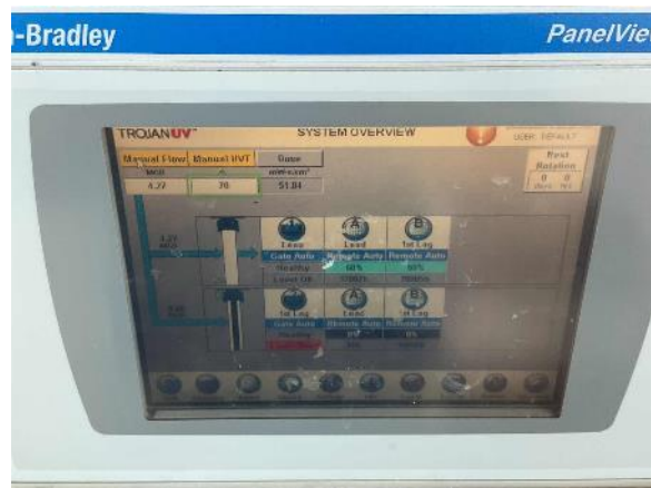
U.V. Bank Control: Pump Station Basement
