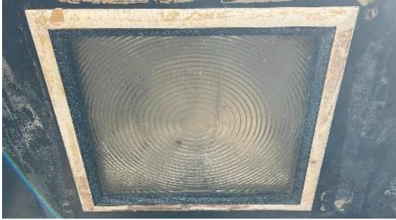
Exterior Incandescent Lamp: Old Admin Building
