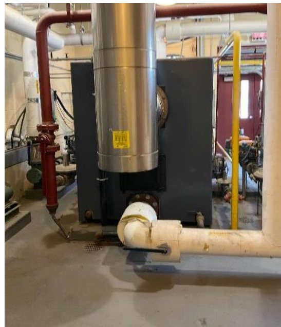
Hydronic Boiler: FMB
