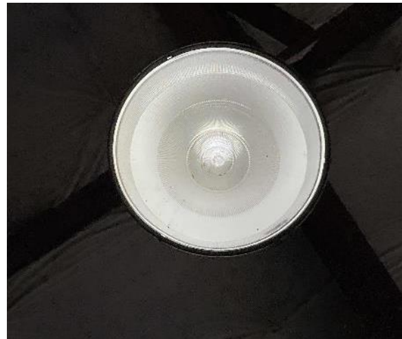
LED High Bay Fixture: Collection Vehicle Garage
