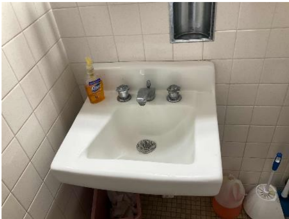
Typical Restroom Faucet: Old Admin Building
