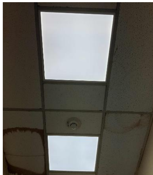
LED 2-foot X 2-foot Fixture: Pump Station
