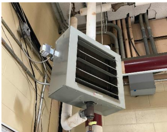
Hot Water Unit Heater: FMB Boiler Room
