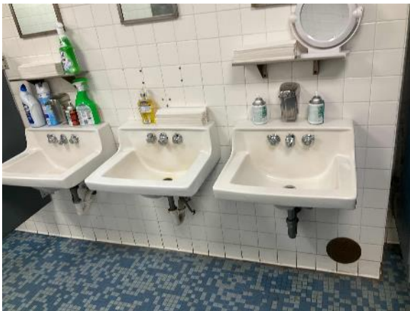
Typical Restroom Faucet: Filter Building
