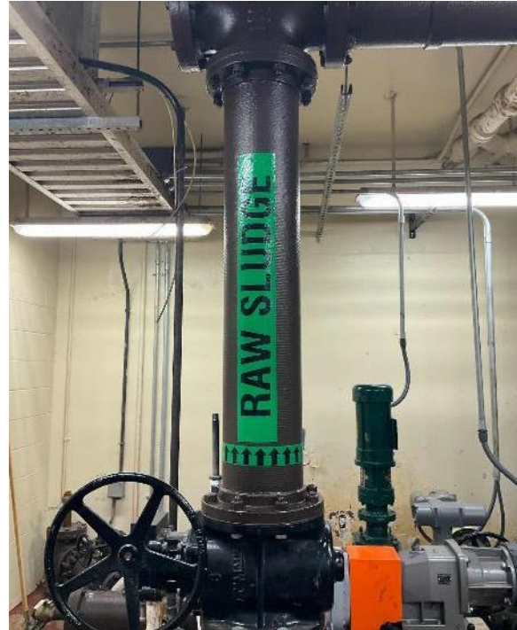
Raw Sludge Pump
