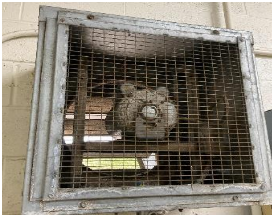
Exhaust Fan: U.V. Disinfection
