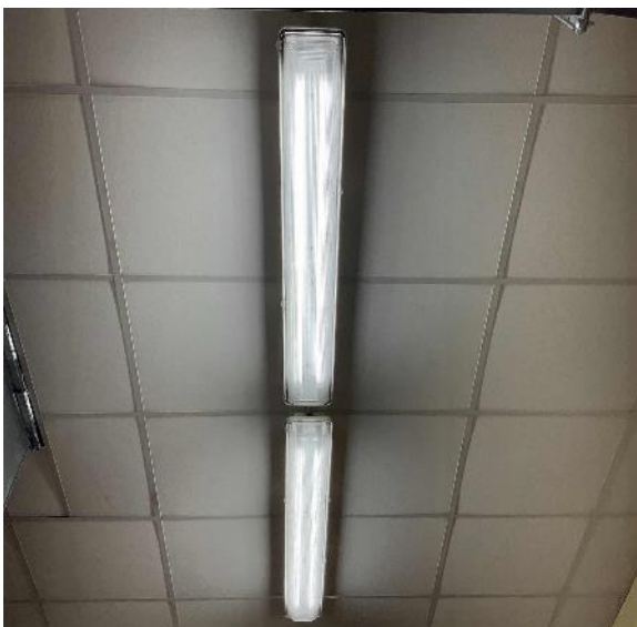
LED Linear Strip: Pump Station
