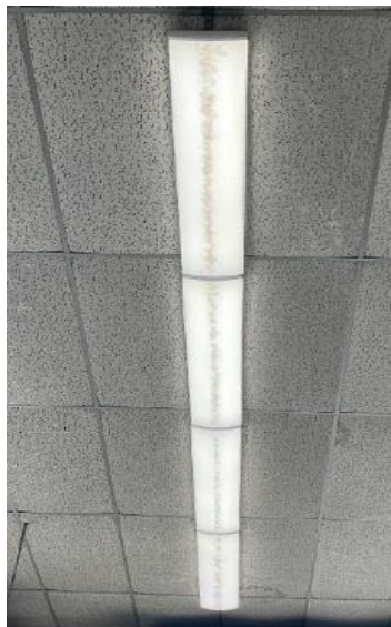
LED Linear Tube: Plant Maintenance Garage
