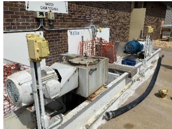
Process Pump: Magnesium Hydroxide Slurry
