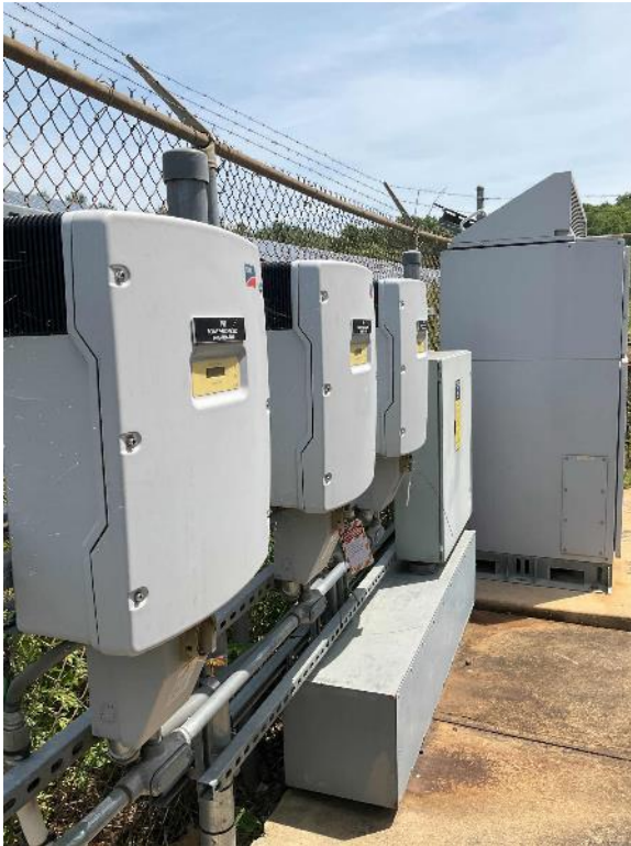
Solar PV Plant: Panel
