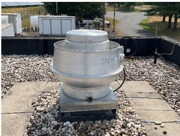
Exhaust Fan: Nitrification Building
