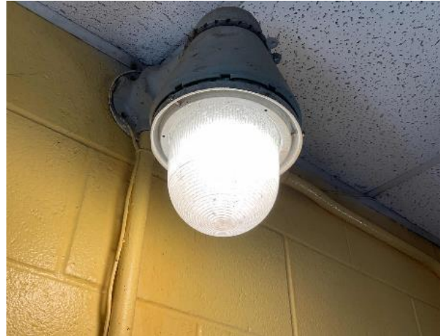
Incandescent Lamp: Digester Building
