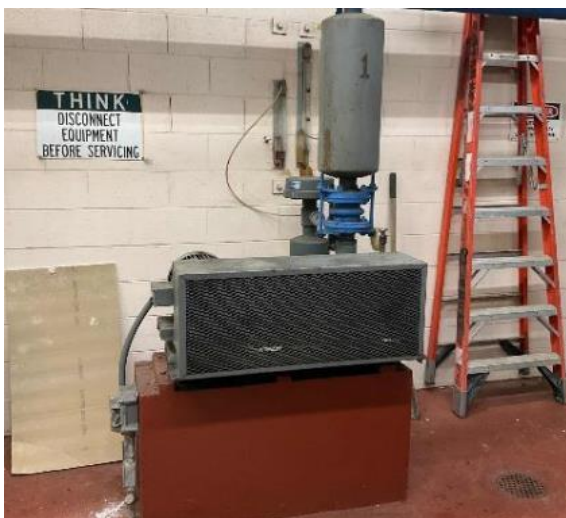
Grit and Screen Blowers
