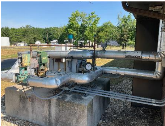
Heat Exchanger: Old Admin Building
