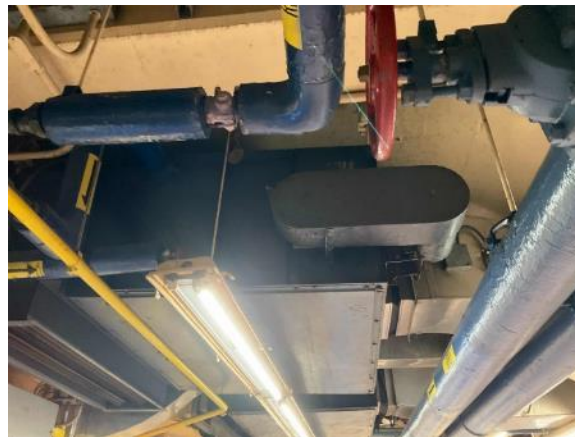
Air Handling Unit: Digester Building
