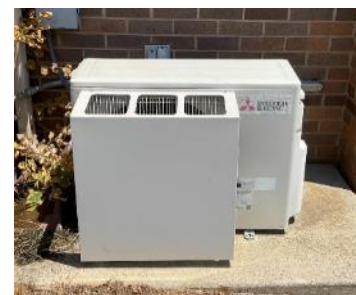
Condensing Unit: Pump Station Control
