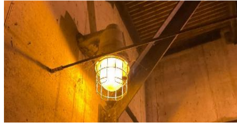
Incandescent Lamp: Pump Station Basement
