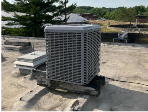
Split Condensing Unit: Filter Building
