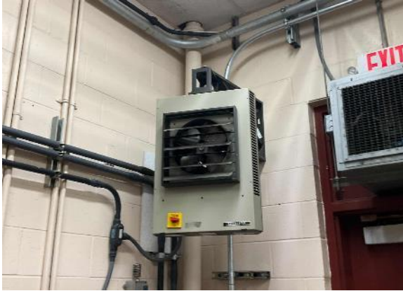
Electric Resistance Heater: Grit Building
