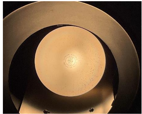
Typical Incandescent Lamp: Old Admin Building
