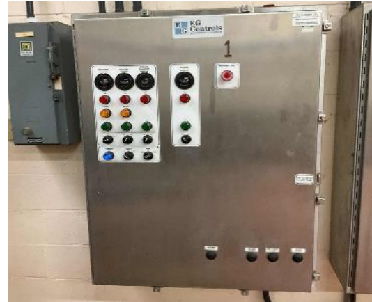
Control Panel: Grit Building
