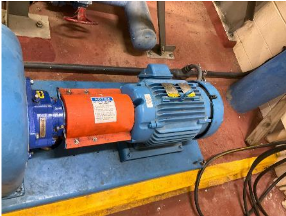
Grit Separation Pump
