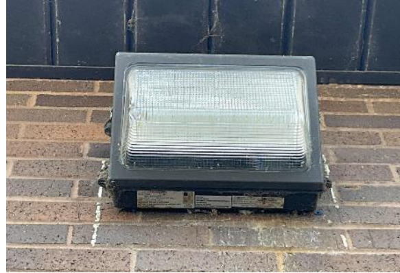
Exterior LED Wall Pack: Plant Maintenance Garage
