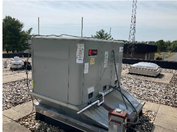
Rooftop Package Unit: Nitrification Building
