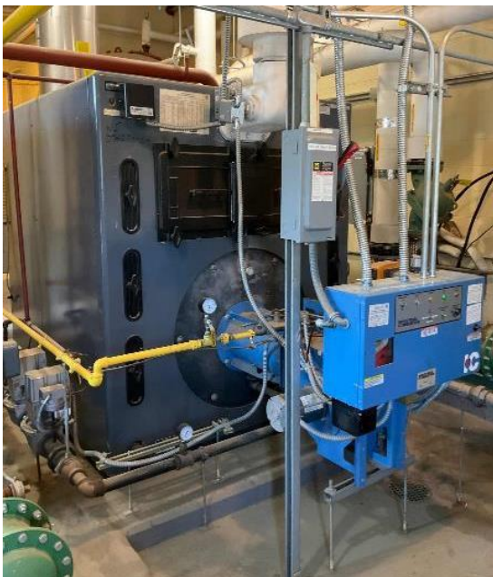
Hydronic Boiler: FMB
