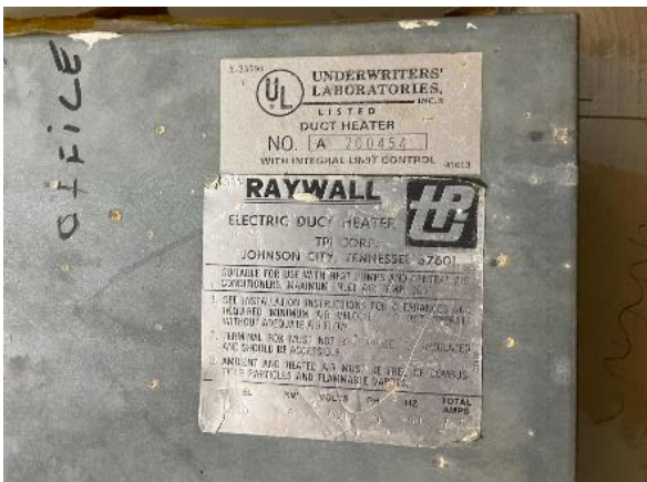
Electric Duct Heater: Old Admin Building
