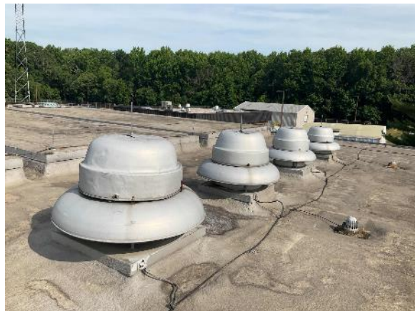
Exhaust Fan: Filter Building
