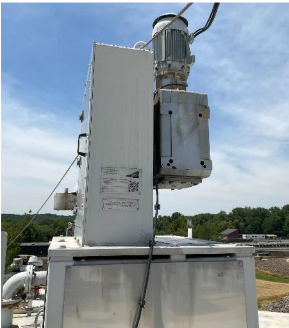
Sludge Mixer: Digester Building
