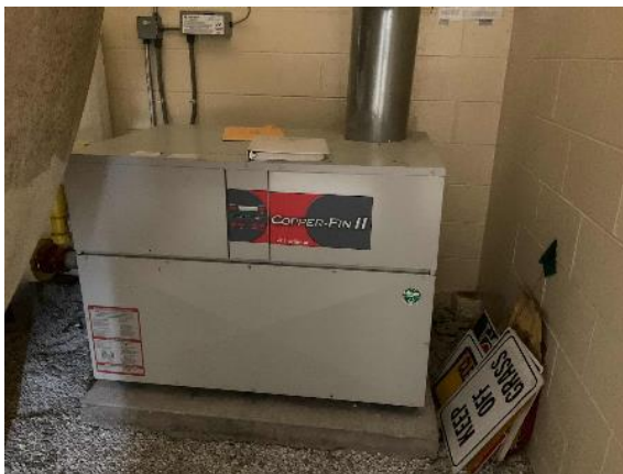
Hydronic Boiler: Filter Building
