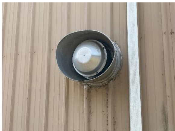
Exhaust Fan: Collection Vehicle Garage
