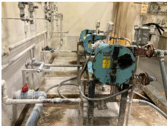
Pump Room: Magnesium Hydroxide Slurry
