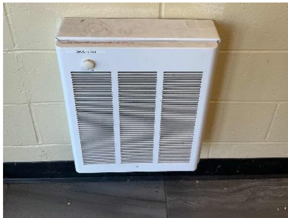
Electric Resistance Heater: FMB Corridor
