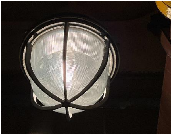
Typical LED Lamp: Digester Building
