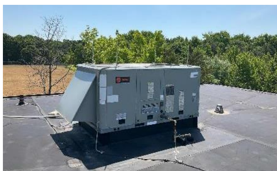
Rooftop Package Unit: FMB
