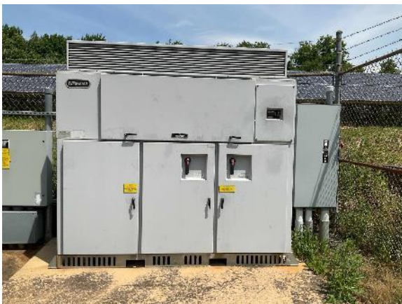
Solar PV Plant: Panel
