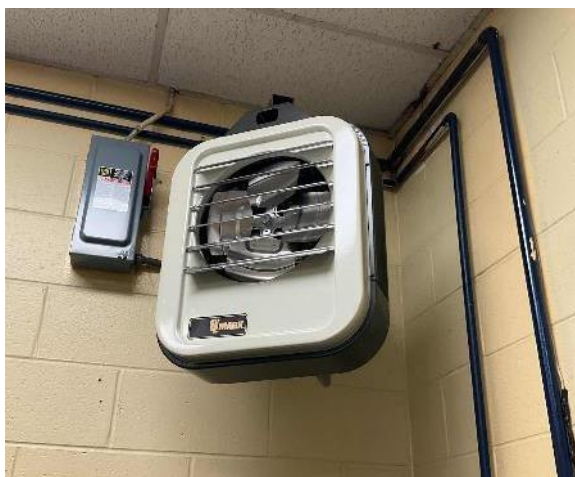
Electric Resistance Heater: Filter Building
