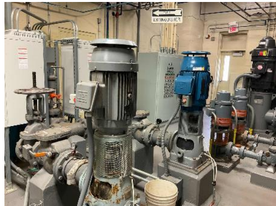
Service Water Pumps
