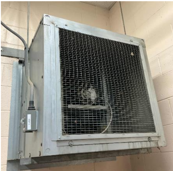
Exhaust Fan: Grit Building
