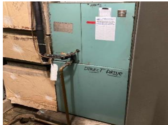
Air Handling Unit: Old Admin Building
