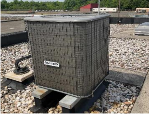
Split Condensing Unit: Nitrification Building
