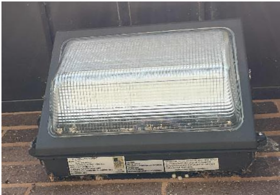
Exterior LED Wall Pack: Digester Building
