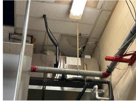
Indoor Air Handler: Filter Building
