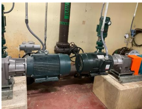
Raw Sludge Pump
