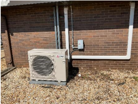
Split Air-Source Heat Pump: Old Admin Building
