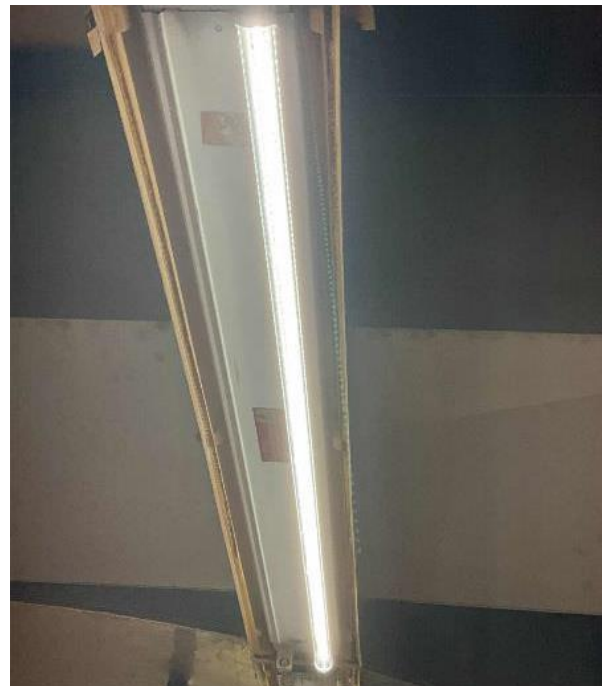
LED Linear Strip: Digester Building
