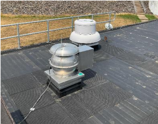
Exhaust Fan: Pump Station
