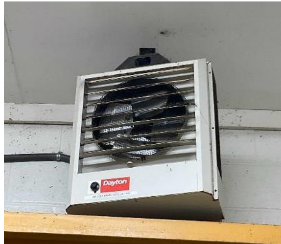
Electric Resistance Heater: U.V. Disinfection
