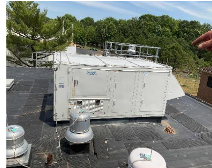
Rooftop Package Unit: Pump Station
