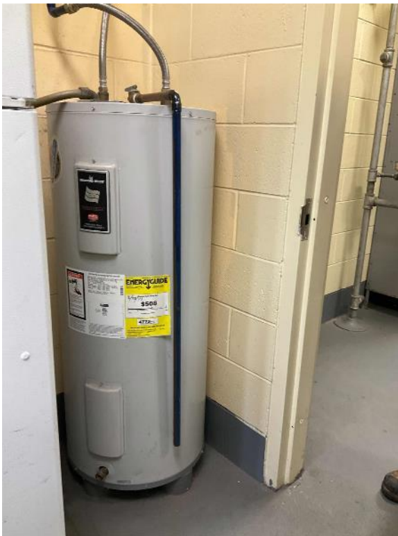
Electric Storage Water Heater: Filter Building
