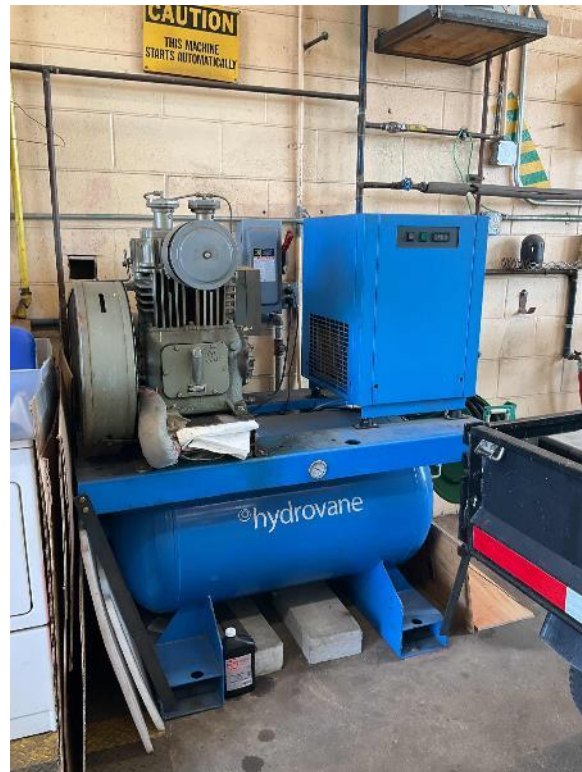
Air Compressor: Plant Maintenance Garage
