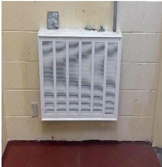
Electric Resistance Heater: Pump Station
