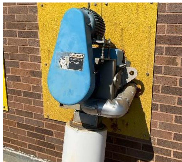
Exterior Grit Pumps
