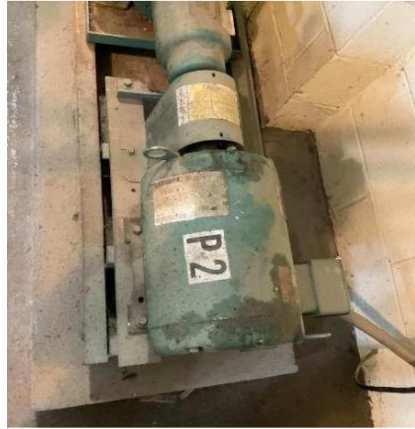
Boiler Heating Hot Water Pump: FMB
