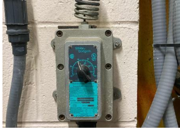
Manual Dial Thermostat: Grit Building
