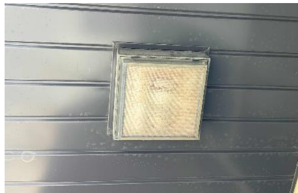
Exterior LED Canopy Fixture: Nitrification Building
