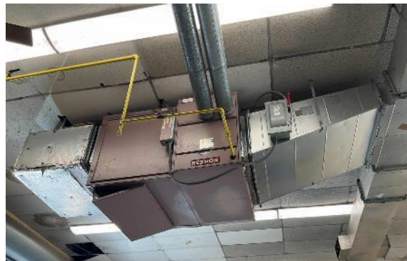
Gas Fired Furnace: Plant Maintenance Garage
