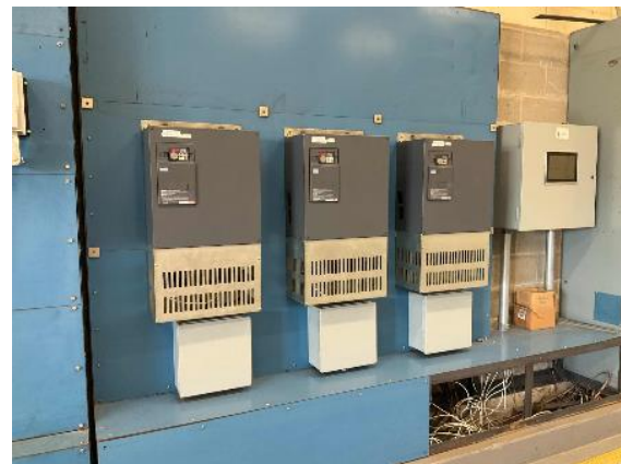
VFD: Sludge Return Pump
