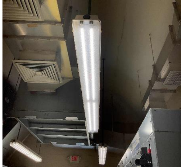
LED Linear Strip: Pump Station Control
