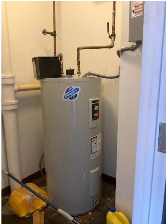
Electric Storage Water Heater: Old Admin Building
