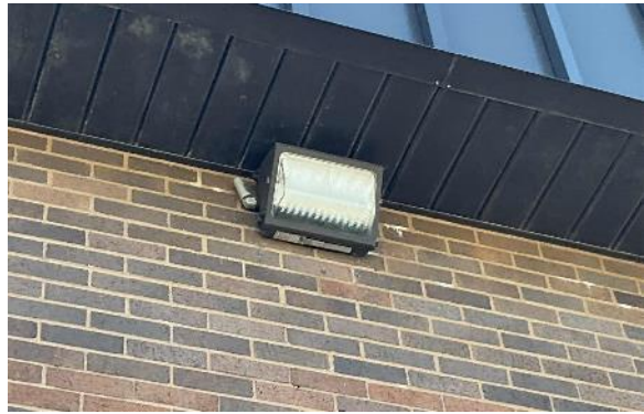
Exterior LED Wall Pack: Grit Building
