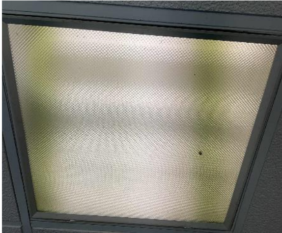
T8 U-Bend Fluorescent: Old Admin Building
