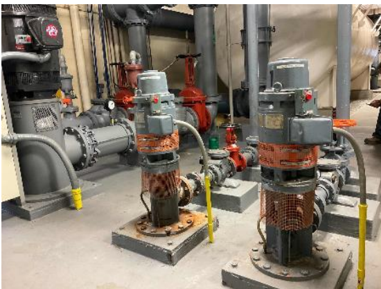
Surface Wash Pumps
