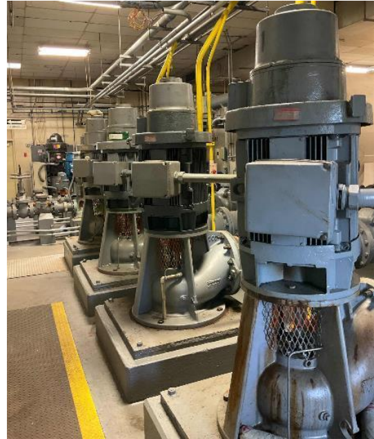
Filter Influent Pumps
