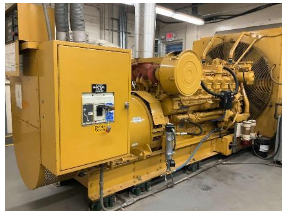
Emergency Generator 910 kW
