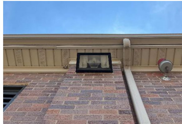
Exterior HID Wall Pack: Pump Station Control
