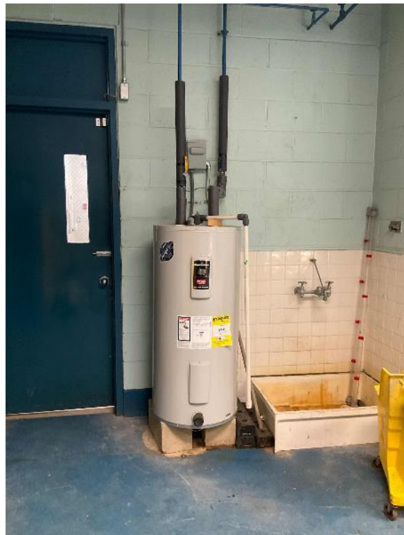
Electric Storage Water Heater: Nitrification Building
