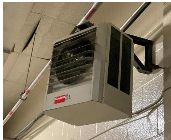
Electric Resistance Heater: Filter Building
