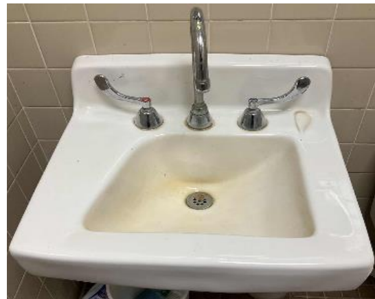
Typical Restroom Faucet: Nitrification Building
