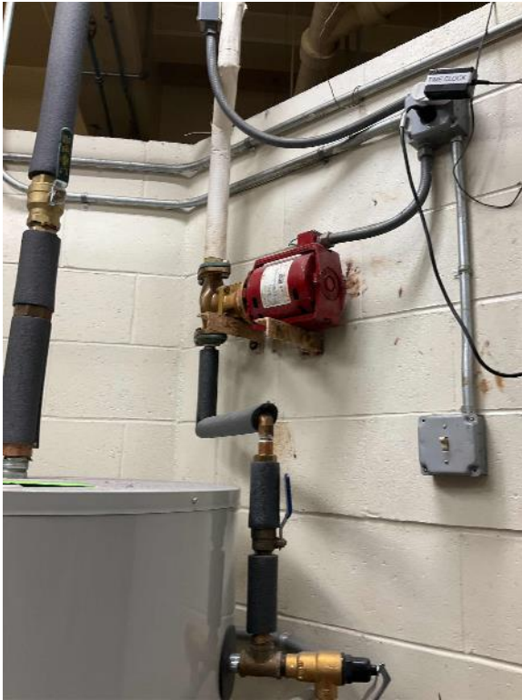
DHW Circulation Pump: FMB
