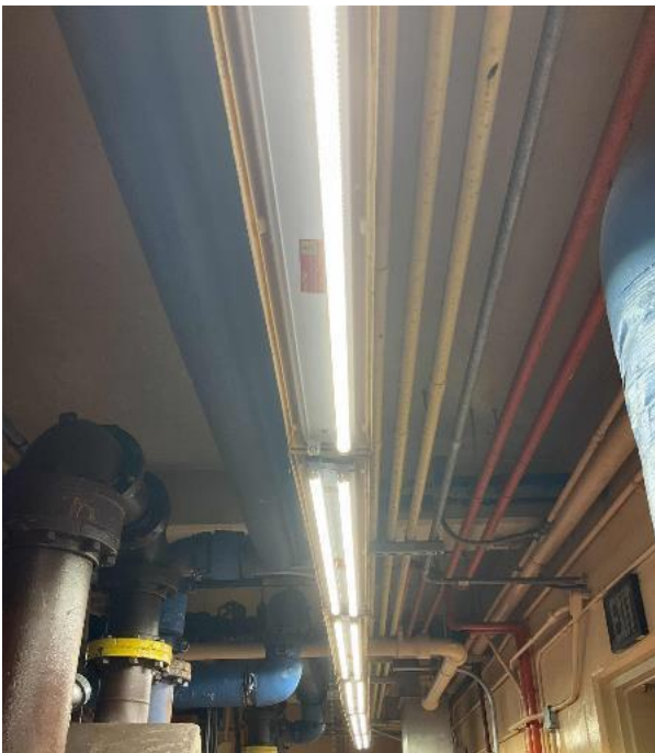
LED Linear Strip: Digester Building
