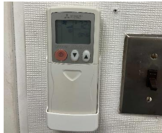
Remote Control: Old Admin Building
