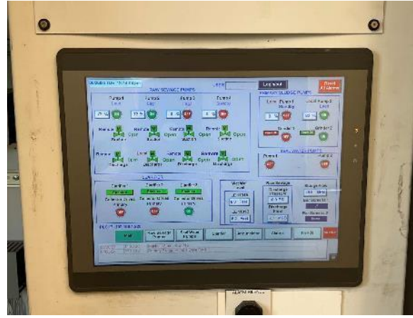
Raw Sewage Pump and Primary Sludge Pump: Control System
