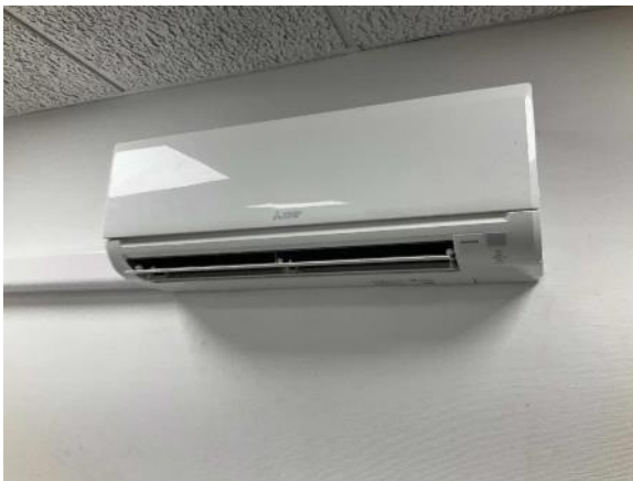
Wall-Mounted Indoor Unit: Old Admin Building
