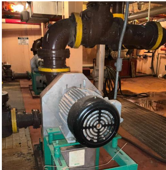
Process Water Pumps
