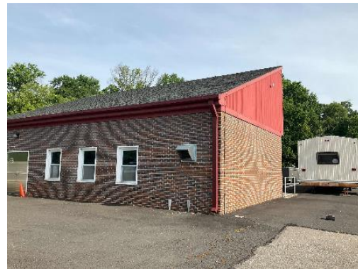
Building Envelope: U.V. Disinfection
