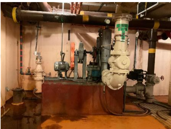
Sludge Pumps: Digester Building
