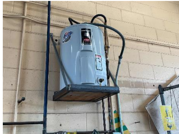
Electric Storage Water Heater: Plant Maintenance Garage
