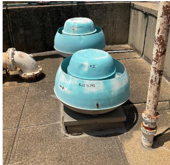
Exhaust Fan: Digester Building
