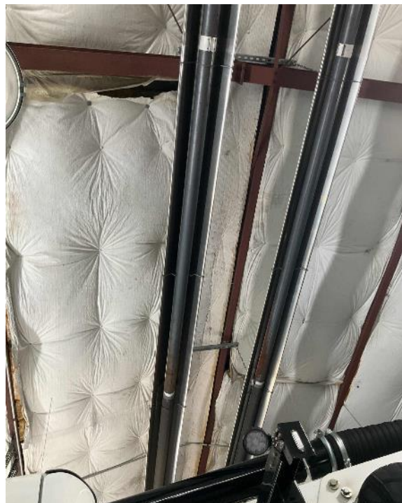
Infrared Heaters: Collection Vehicle Garage
