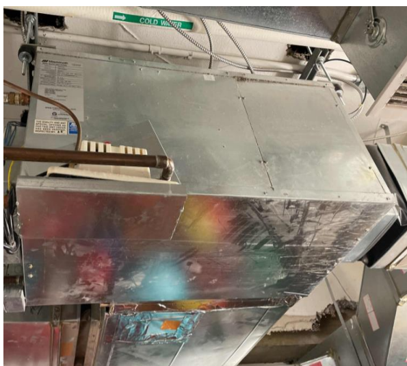
Gymnasium Water Source Heat Pump
