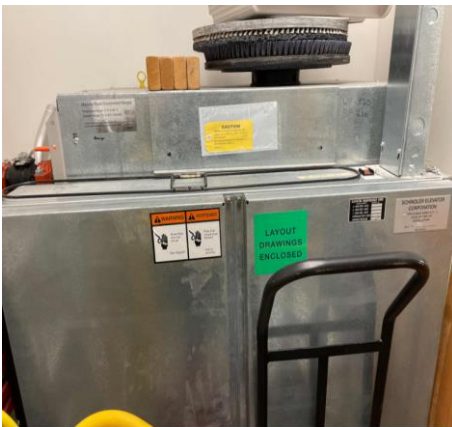
Elevator Hydraulic Pump
