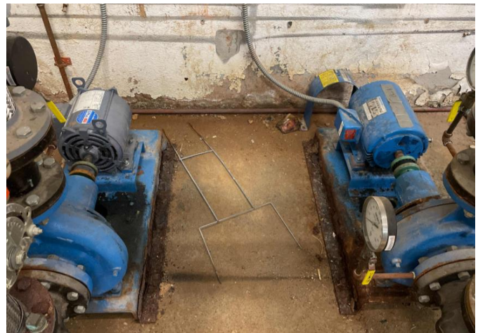
Heating Hot Water Pumps
