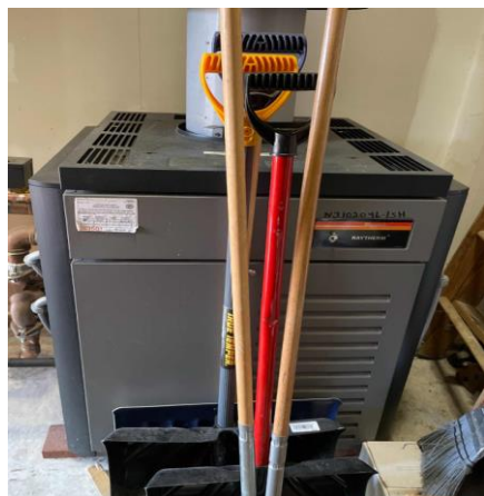
Domestic Hot Water Heater
