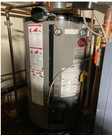
Domestic Hot Water Heater
