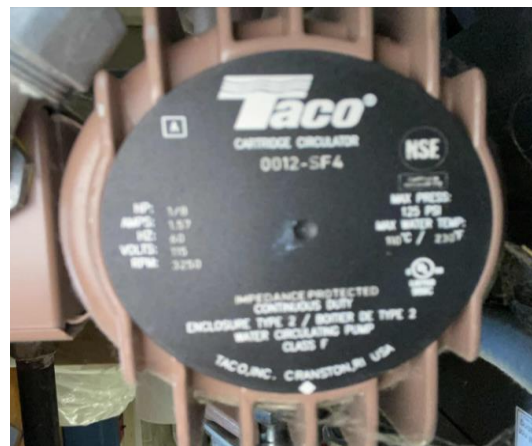
DHW Circulation Pump
