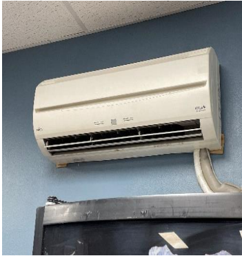
Ductless Mini-split Unit
