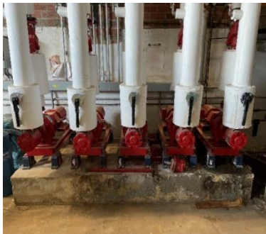
Heating Hot Water Pumps
