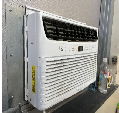
Window AC Unit
