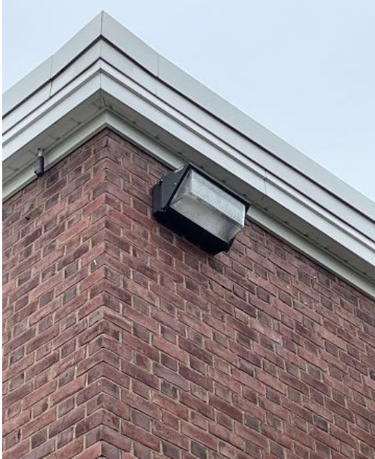
Exterior Metal Halide Fixtures
