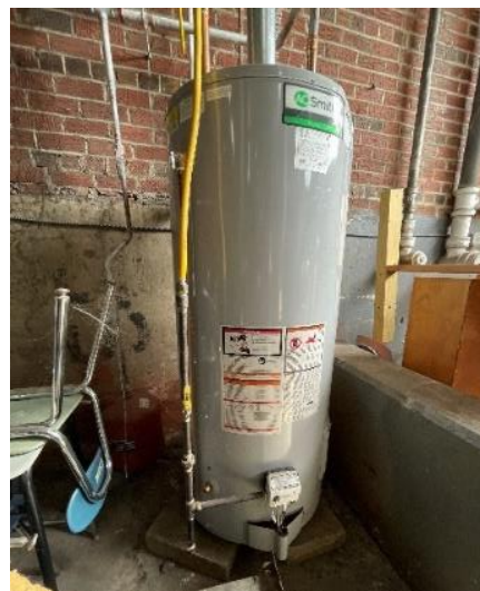
Domestic Hot Water Heater
