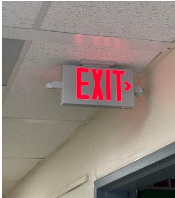
LED Exit Signs
