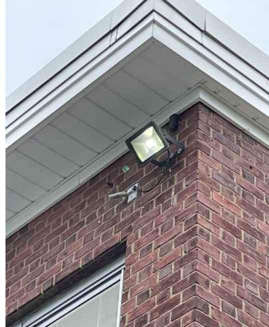
Exterior LED Fixtures
