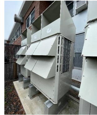
VRF Heat Pump Units
