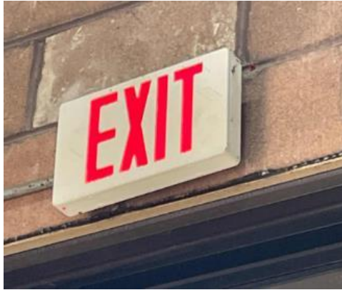
Incandescent Exit Sign
