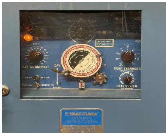
Steam Boiler Controls
