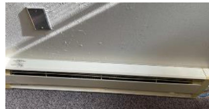
Electric Resistance Heater
