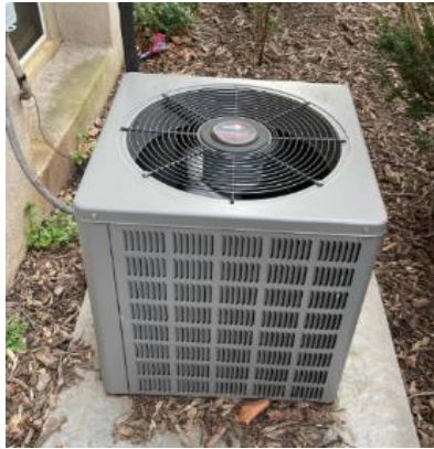
Split system AC unit
