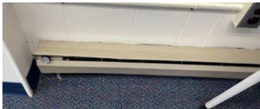
Electric Resistance Heater
