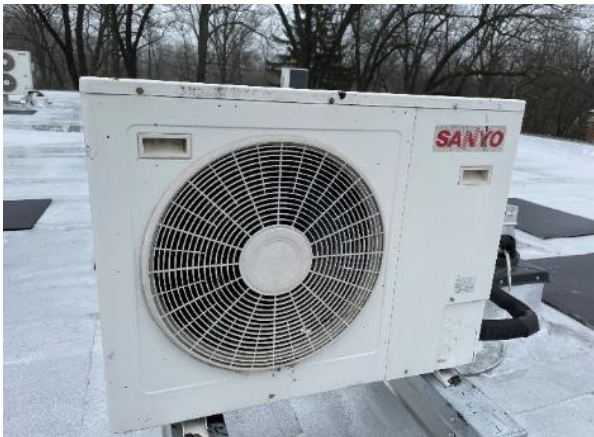
Outdoor Condensing Unit
