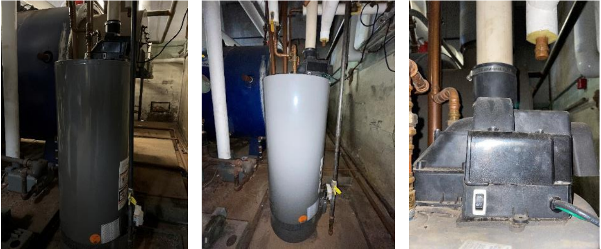
Storage Water Heater
