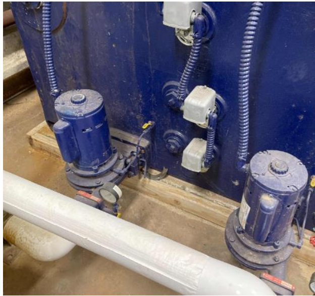
Heating Hot Water Pumps
