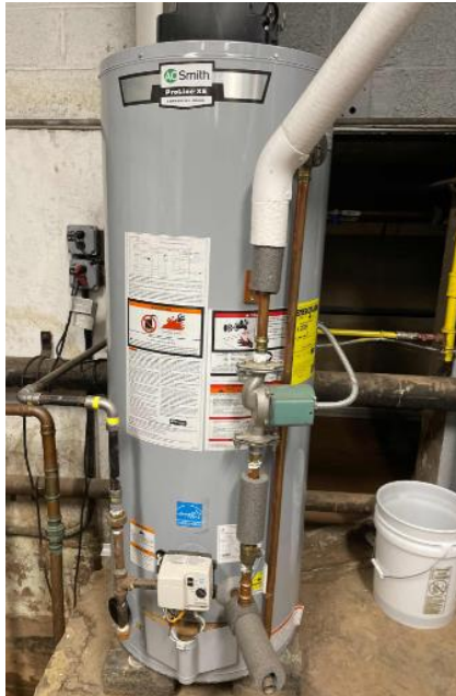
Domestic Hot Water Heater
