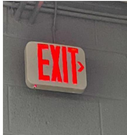
LED Exit Sign
