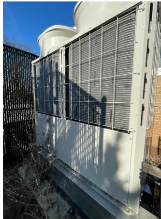
Variable Refrigerant Flow
