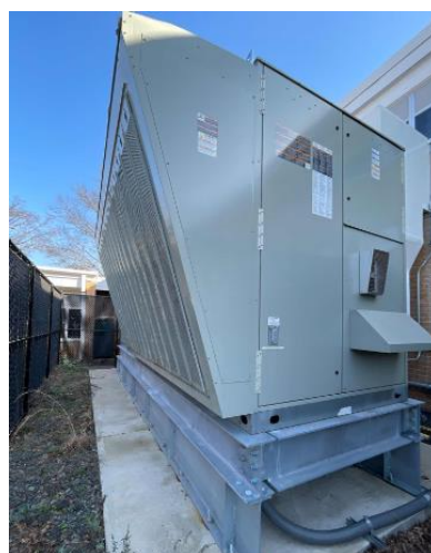
Outdoor Air Unit
