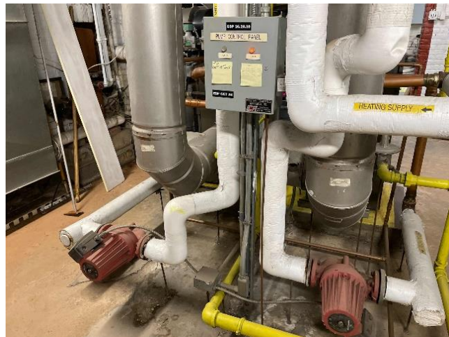
DHW Circulation Pumps and Controls
