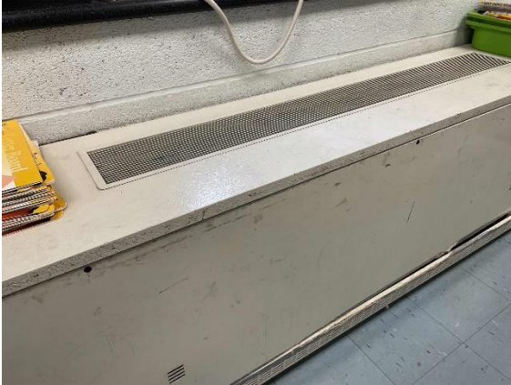
Classroom Unit Ventilator
