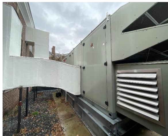
Package Unit Ducting
