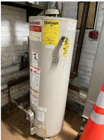
Natural Gas DHW Heater
