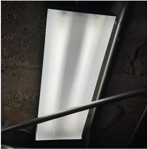
Linear Fluorescent – Storage Room
