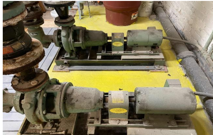
HHW Circulation Pumps
