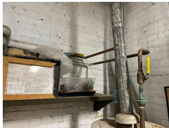
Uninsulated DHW Pipes – Natural Gas Unit
