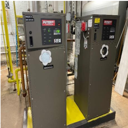
HHW Boilers – Boilers #1 and #2
