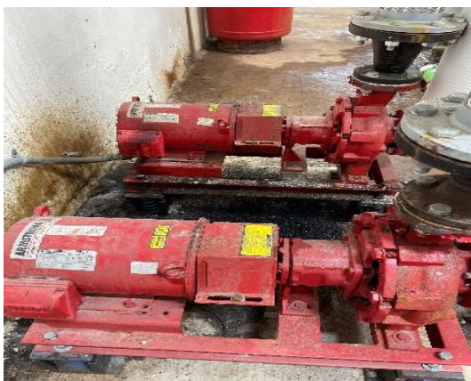
HHW Circulation Pumps
