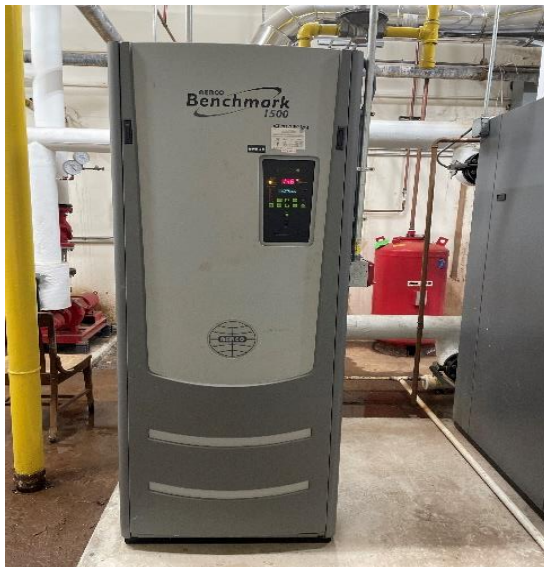
Condensing HHW Boiler
