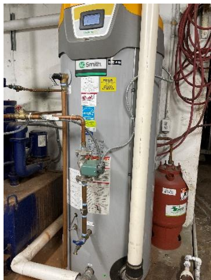
Condensing Hot Water Heater
