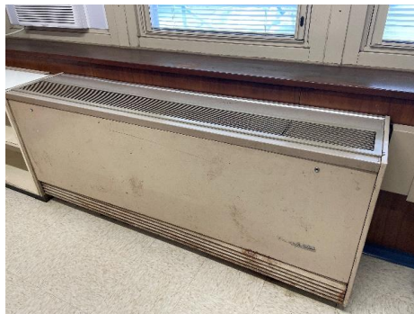
Classroom Unit Ventilator
