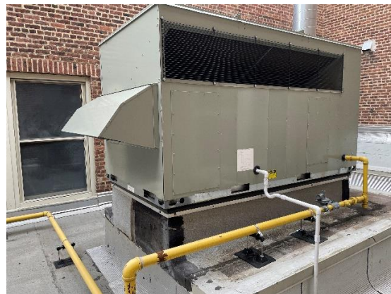
Trane Packaged Unit
