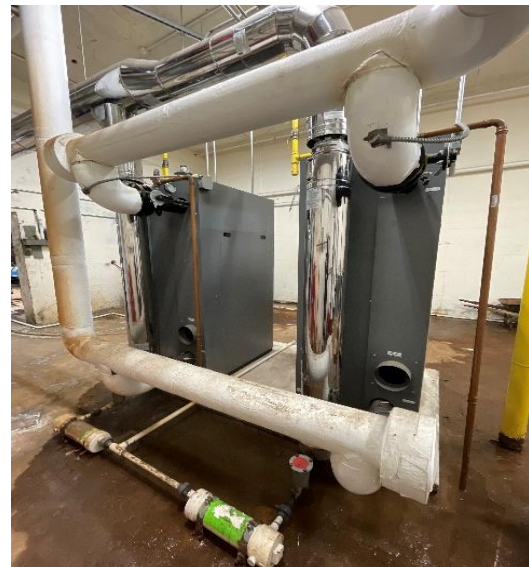
HHW Boilers and Pipe Insulation
