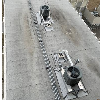
Inaccessible Condensing Unit
