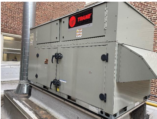
Trane Packaged Unit
