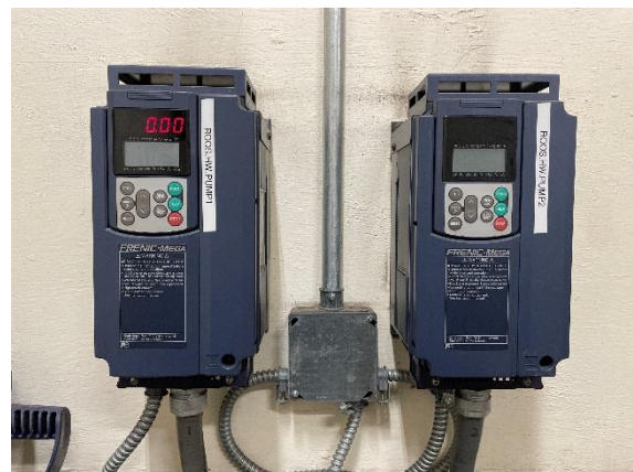
HHW Pump VFDs
