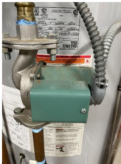
DHW Circulation Pump
