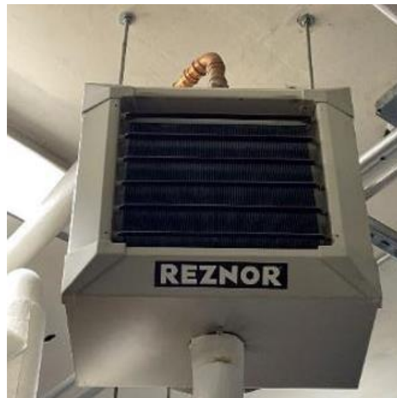
Boiler Room Heater
