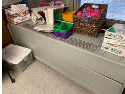
Classroom Unit Ventilator
