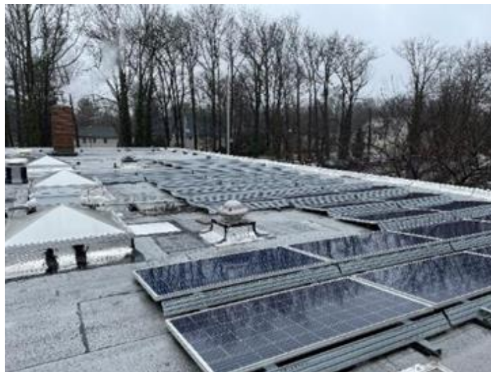
Roof Solar Panel Array
