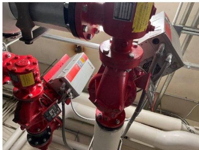
HHW Pumps and VFDs
