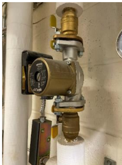
DHW Circulation Pump
