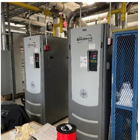
Condensing HHW Boilers
