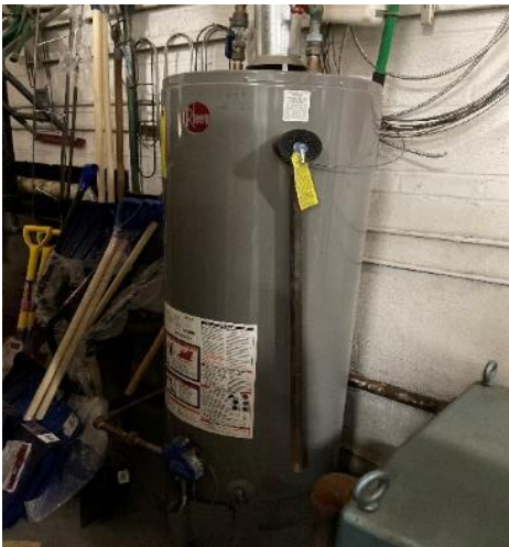
Hot Water Storage Tank
