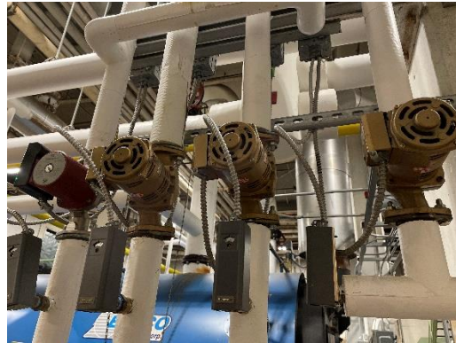
DHW Circulation Pumps
