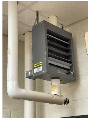
HHW Unit Heater
