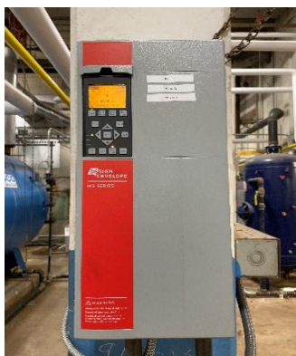
HHW Pump VFD
