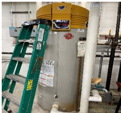
2002 Condensing Hot Water Heater
