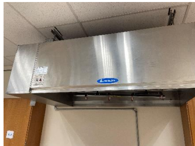
Kitchen Fume Hood–Classroom
