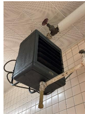
HHW Unit Heater— Uninsulated Return Pipe
