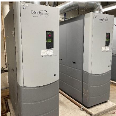
Condensing HHW Boiler
