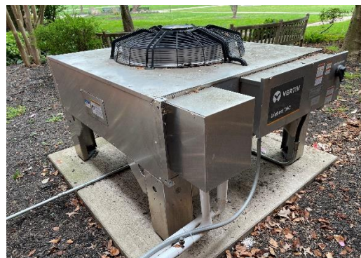
CRAC Condensing Unit
