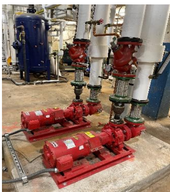
HHW Pumps with VFDs
