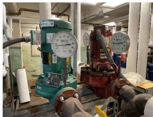
HHW Pumps no VFD
