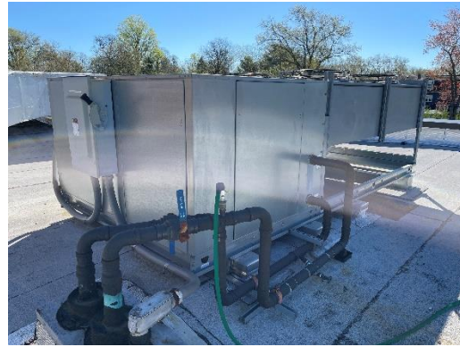
CRAC Condensing Unit
