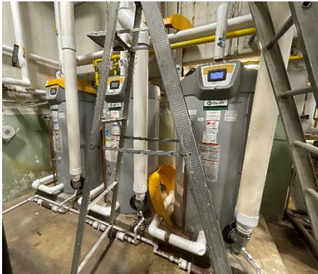
Condensing Hot Water Heaters
