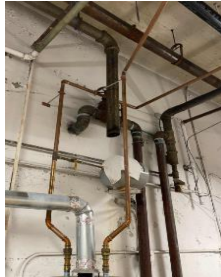
Uninsulated DHW Pipes
