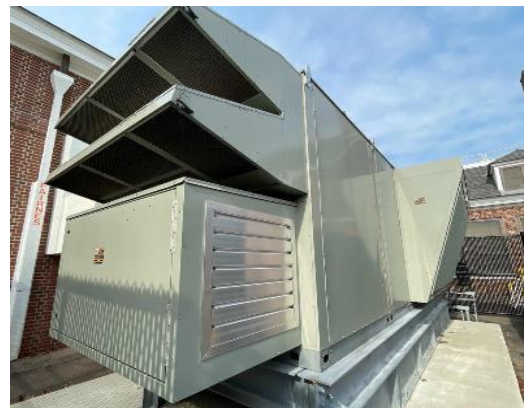
Outdoor Air Unit
