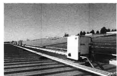
5 SMA STRING INVERTER
