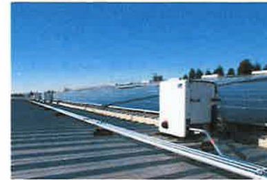
3 SMA STRING INVERTER SCALE SITE
