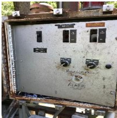
Pump Control Panel
