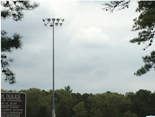
Pole Fixture with 9 Lamps
