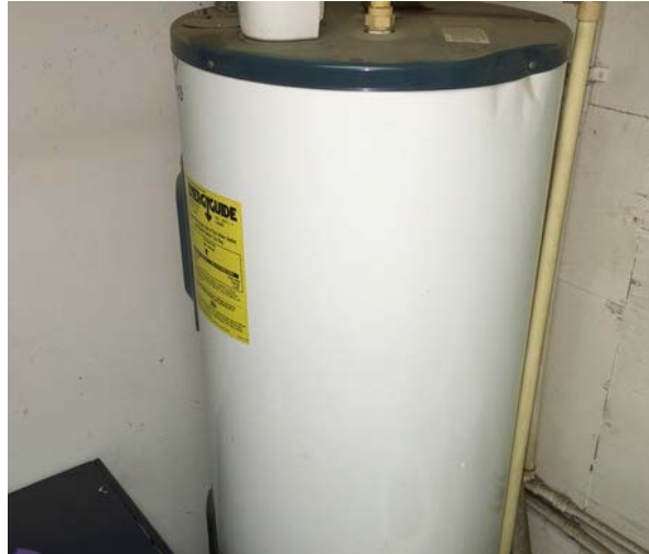
Domestic Hot Water Heater
