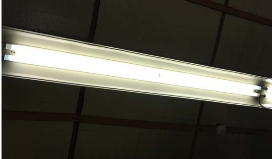
8 Ft T12 Fixture
