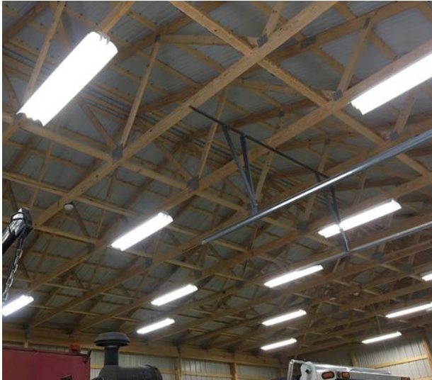
2 Lamp T8 Fixtures
