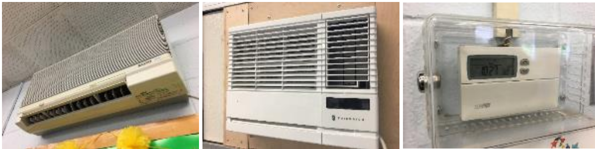
Image 5 Direct Expansion AC system
