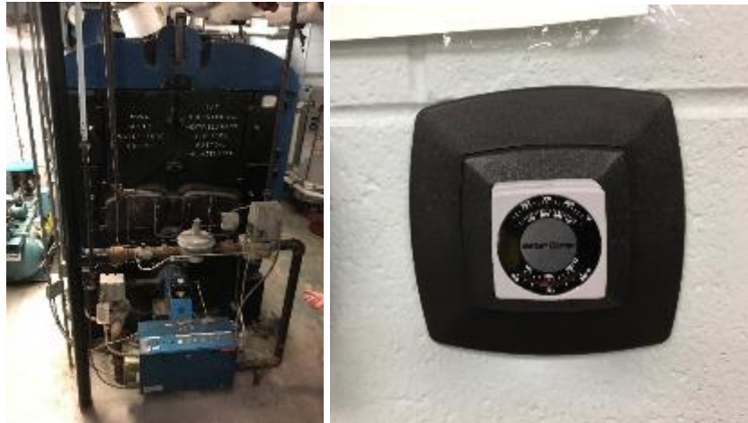
Image 3 Hot water heating system
