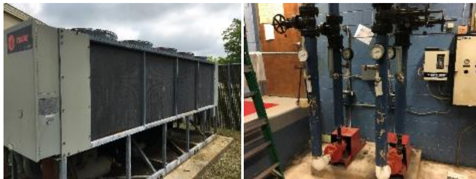
Image 4 Chilled Water System
