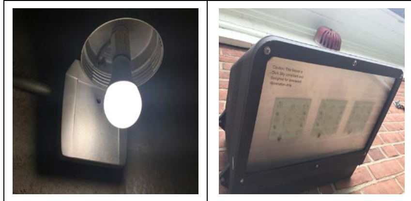
Image 3: Interior & Exterior Lighting System
