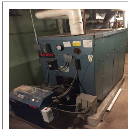
Image 4: Smith Hot Water Boiler
