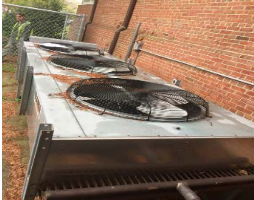
Image 6: Air-Cooled Condensing Unit (Split AC)
