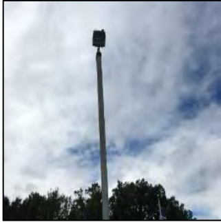
Pole Light Fixtures
