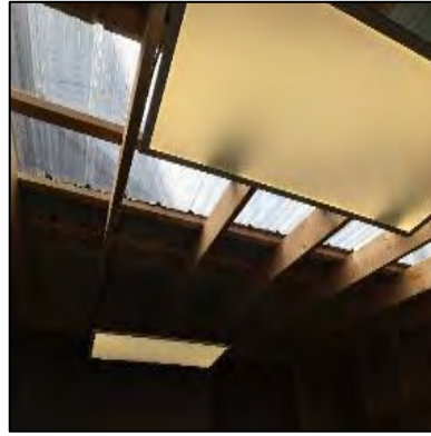
Testing Room LED Panels
