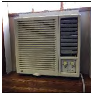
Office Window AC
