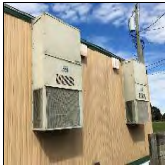
Packaged Terminal Heat Pumps (#1 & #2)
