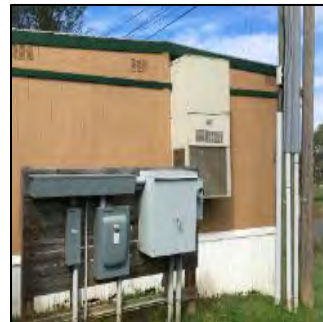
Packaged Terminal Heat Pump (#3)
