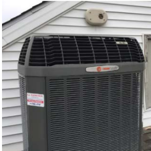
Outdoor Trane AC Unit
