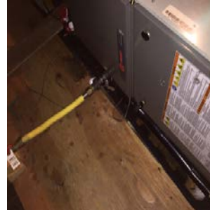
Gas-fired Heating serving the package unit
