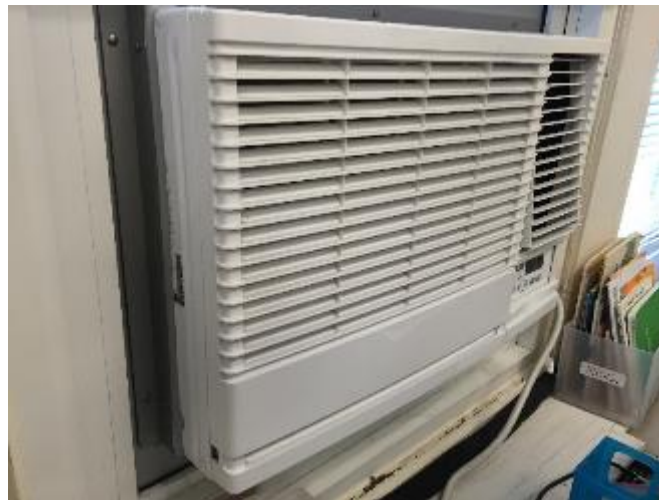
AC Window Unit
